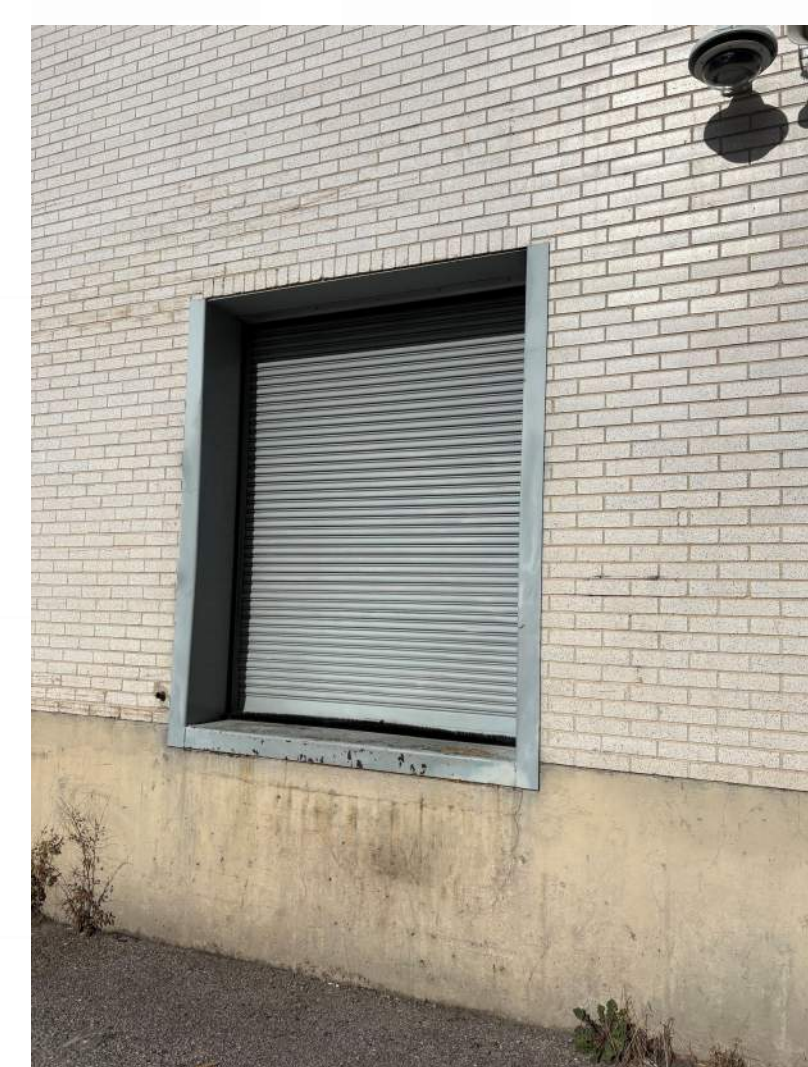
EXISTING OVERHEAD DOOR TO BE REPLACED WITH DOUBLE DOORS. OPENING WILL BE LOWERED TO ALLEY LEVEL.
