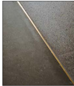
Metal inlay between stained concrete and exposed aggregate paving
