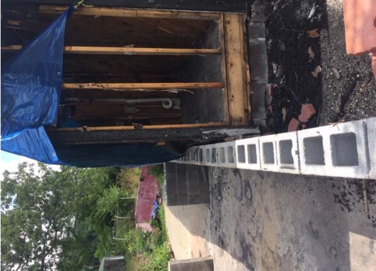
Existing conditions, fire damaged structure.
