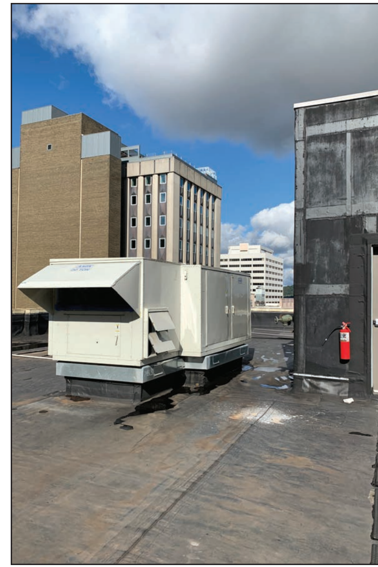
EXISTING ROOFTOP LOOKING NORTH AT ERV
