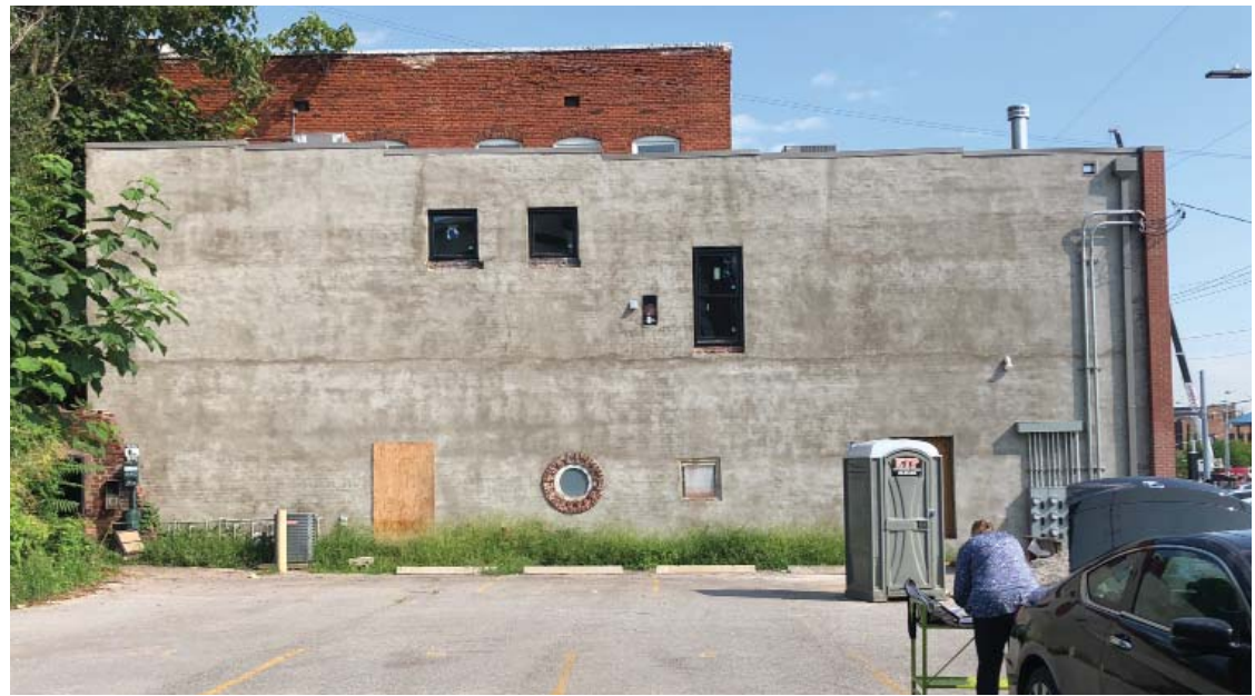
View Northwest from Adjacent Lot: Existing Conditions Addition to be located along South elevation of the existing building.
