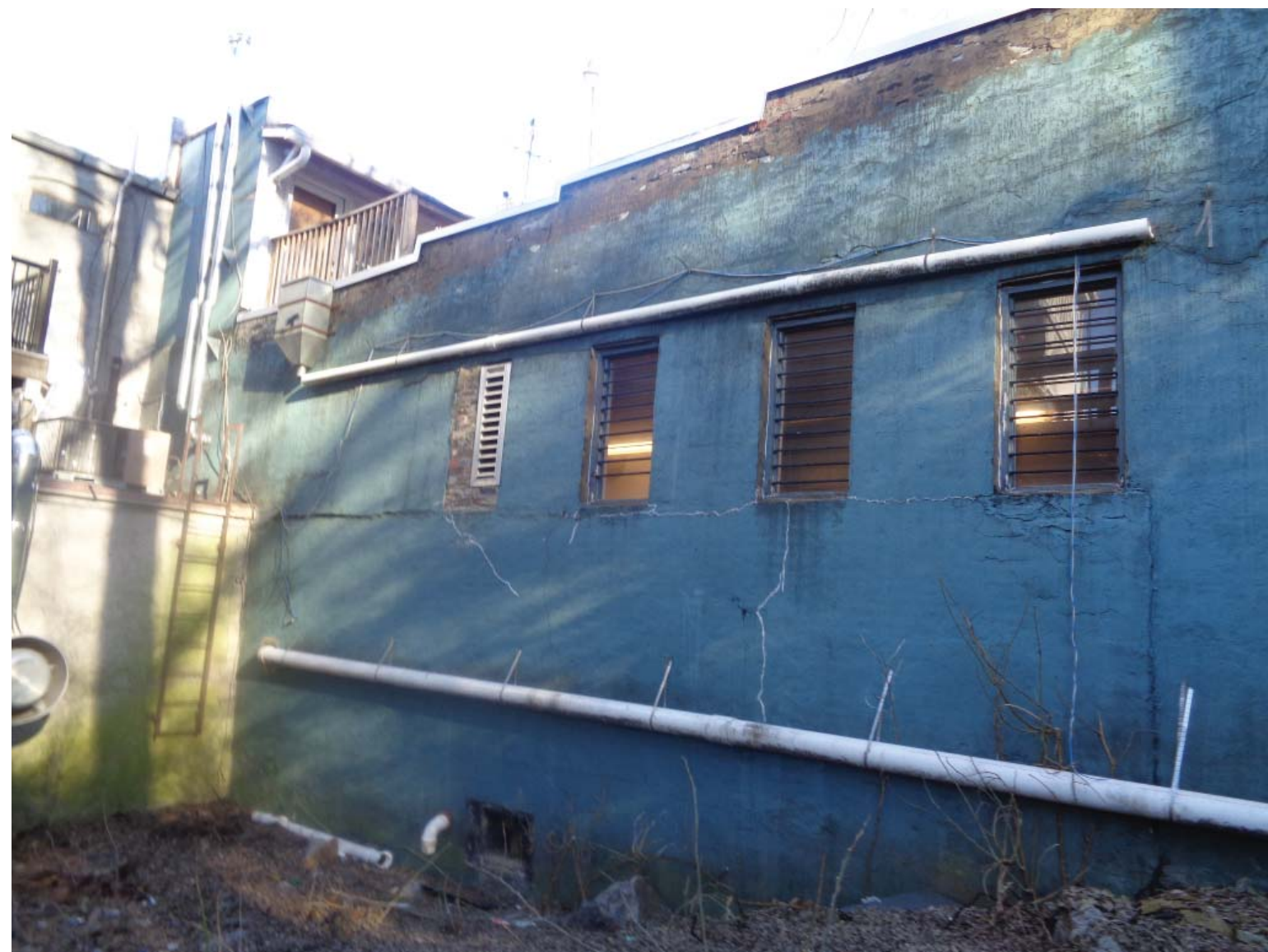
NORTH WALL OF STORAGE ROOM. SCOPE INCLUDES REMEDIAL STRUCTURAL WORK. (OR REPLACEMENT OF WALL)
