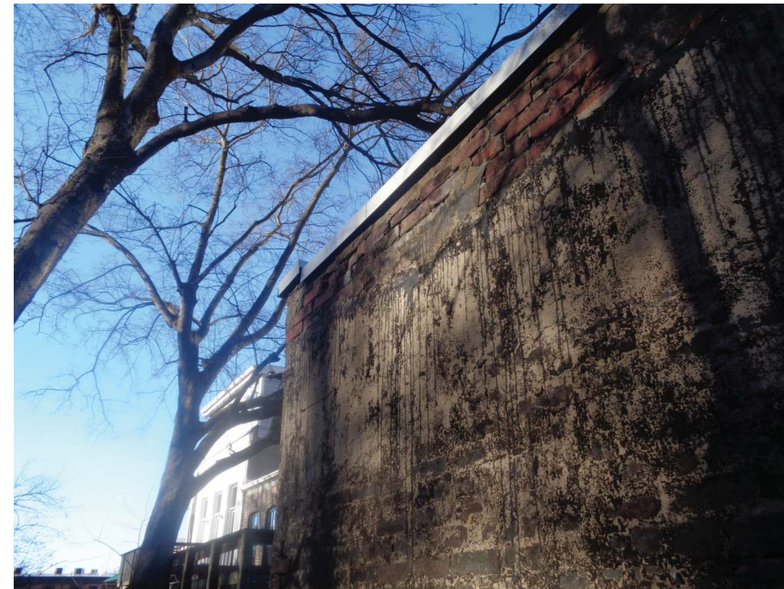
EXISTING WEST WALL OF STORAGE ROOM - BRICK JOINTS WILL BE REPOINTED AS REQ.
