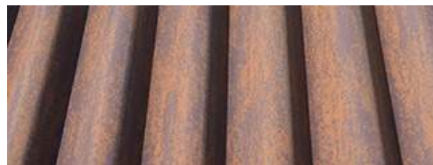
PAINTED RUSTED ROOFING
