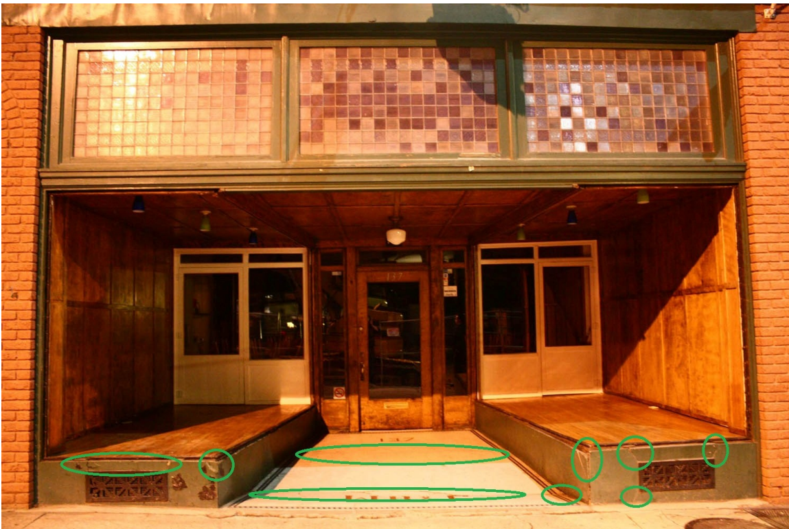
STOREFRONT DAMAGE LOCATIONS
