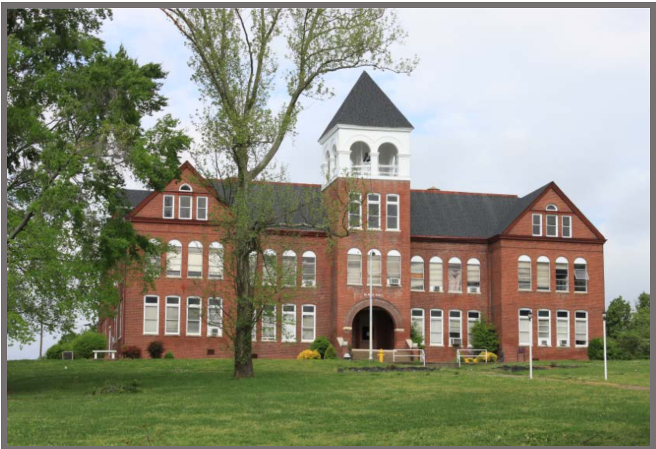
The roof and supporting wall on the rear of the 1876 McKee Hall Administration Building have collapsed.
