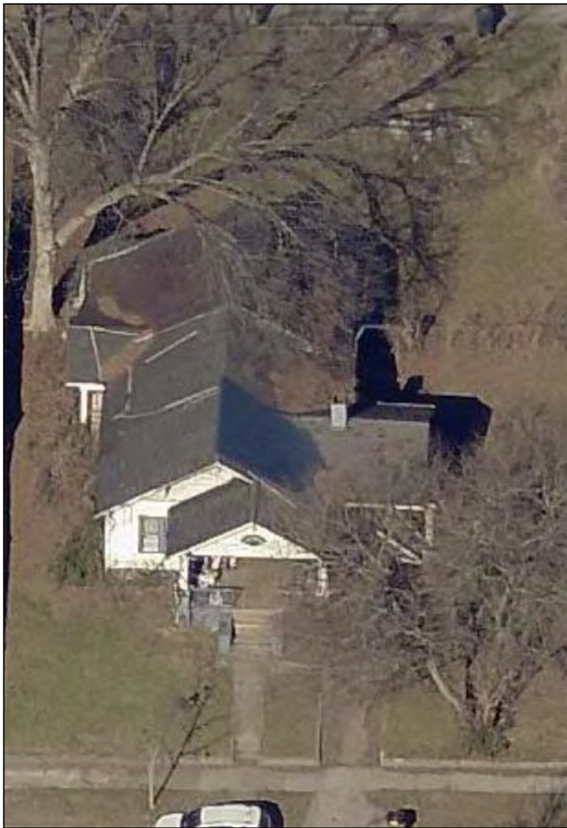
KGIS Pictometry, February 2024 Front porch supports and chimney
