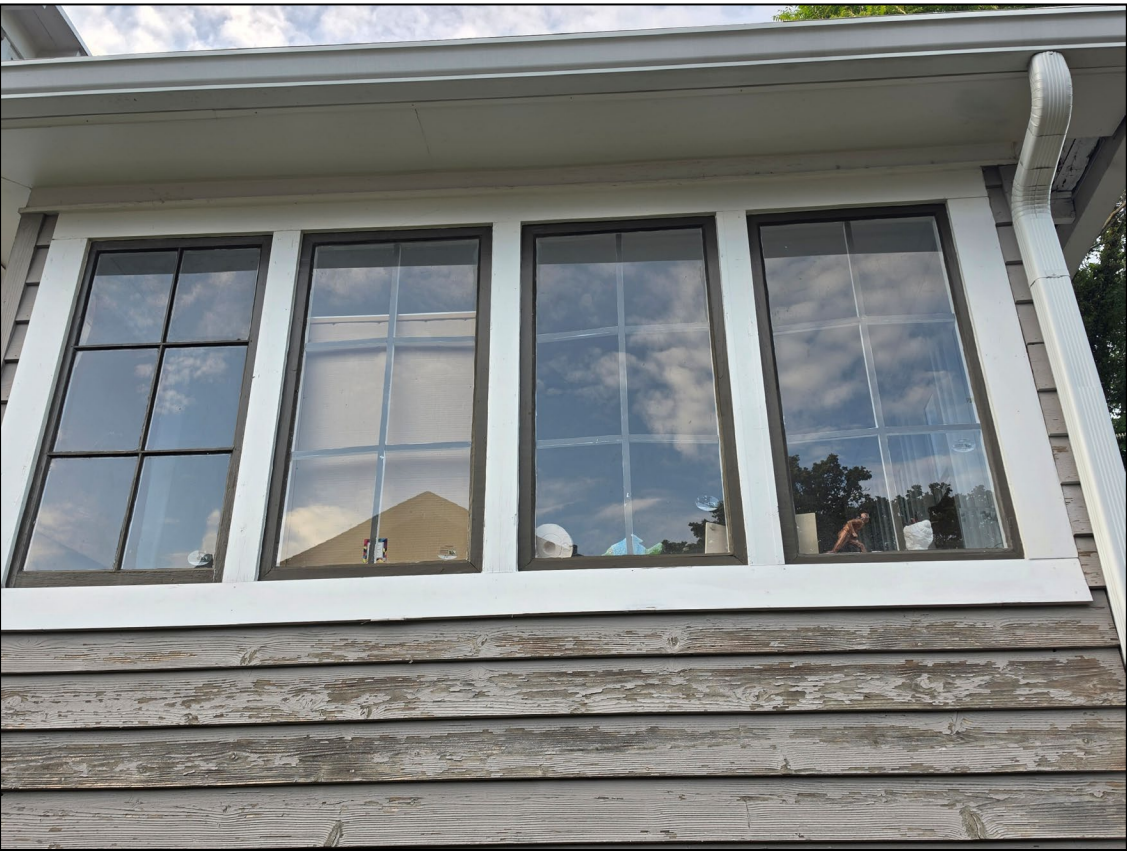
Three non-historic windows in office (south elevation)
