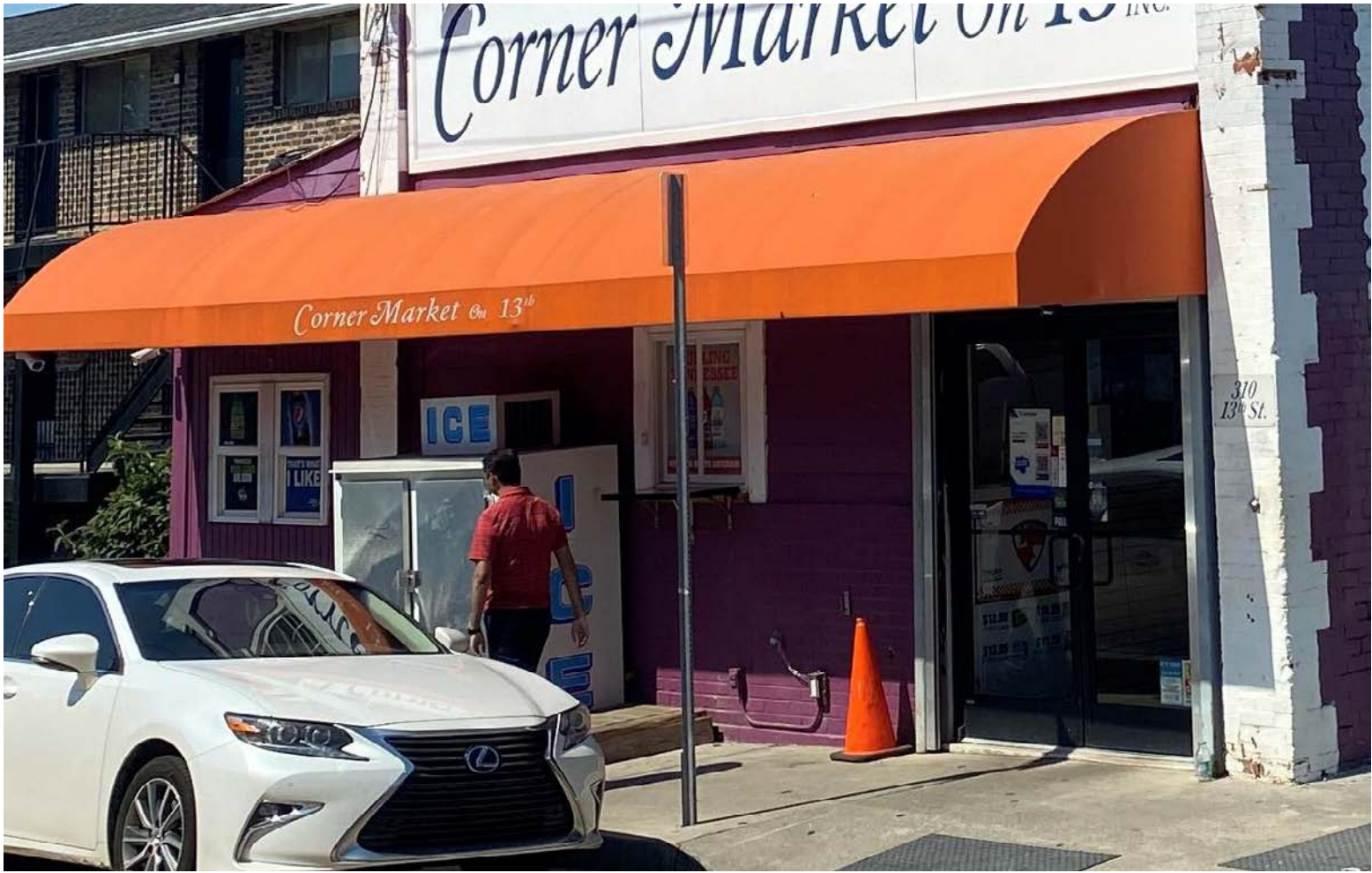
View of the front facade where the storefront has been filled in with siding, walkup window, and door.
