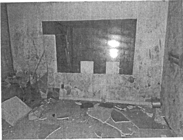
43. West Side of Basement. Moisture Intrusion, Mold.
