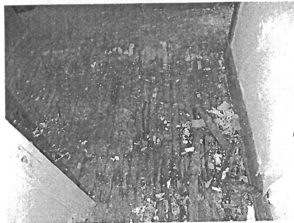
32. Side Room, Southwest Corner of Building. Water Damage, Rotted Flooring, Mold.
