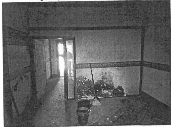
23. Side Room, East Side of Building. Water Damage, Mold.
