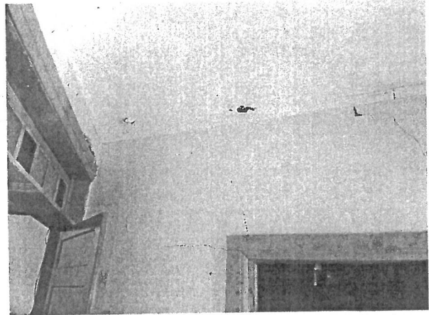
28. Side Room, Northeast Corner of Building. Water Damage, Mold, Settlement Cracks.
