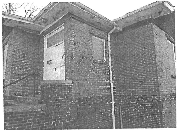
4. Northwest Corner. Mismatched Brickwork, Deteriorated Mortar, Brick Pulling from Wall, Missing Brick, Damaged Soffit, Poor Flashing.
