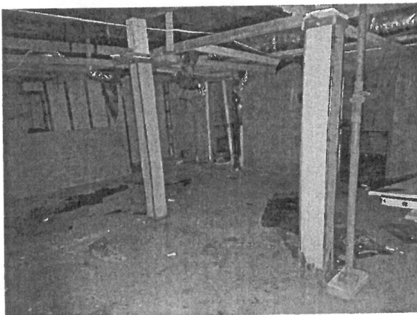
33. Basement, Central Room. Rotted Support Posts, Mold.
