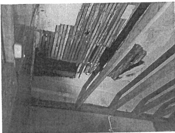
21. Side Room, East Side of Building. Water Damage, Rotted Roof Joists, Mold.
