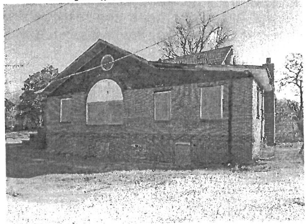
5. West Side. Damaged Soffit, Delaminated Shingle Veneer, Poor Flashing, Missing Brick, Brick Pulling from Building Wall.
