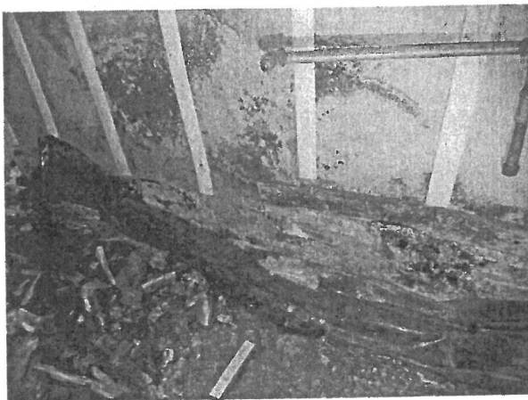
39. East Side of Basement. Moisture Intrusion, Mold.
