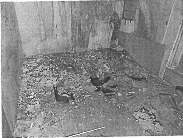
19. Side Room, Southeast Corner of Building. Water Damage, Rotted Floor, Mold.
