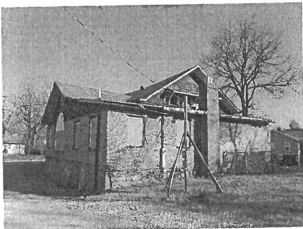
9. Rear (South Side). Missing Window, Patched Brick, Damaged Soffit & Rafters, Delaminated Shingle Veneer, Missing Brick, Brick Pulling from Building Wall.
