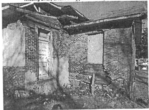
12. Southeast Corner. Patched Brick, Damaged Soffit & Rafters, Delaminated Shingle Veneer, Missing Brick, Brick Collapse, Damaged Wall Sheathing.
