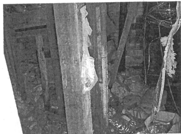
36. South Side of Basement. Rotted Support Posts, Rotted Stud Walls, Moisture Intrusion, Mold.
