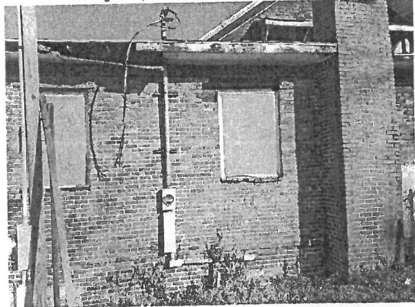
11. Rear (South Side). Missing Window, Patched Brick, Damaged Soffit & Rafters, Delaminated Shingle Veneer, Missing Brick, Brick Pulling from Building Wall.
