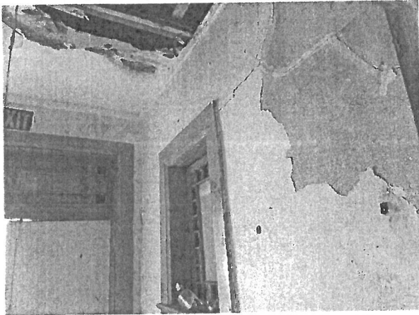
26. Side Room, Northeast Corner of Building. Water Damage, Mold, Settlement Cracks.
