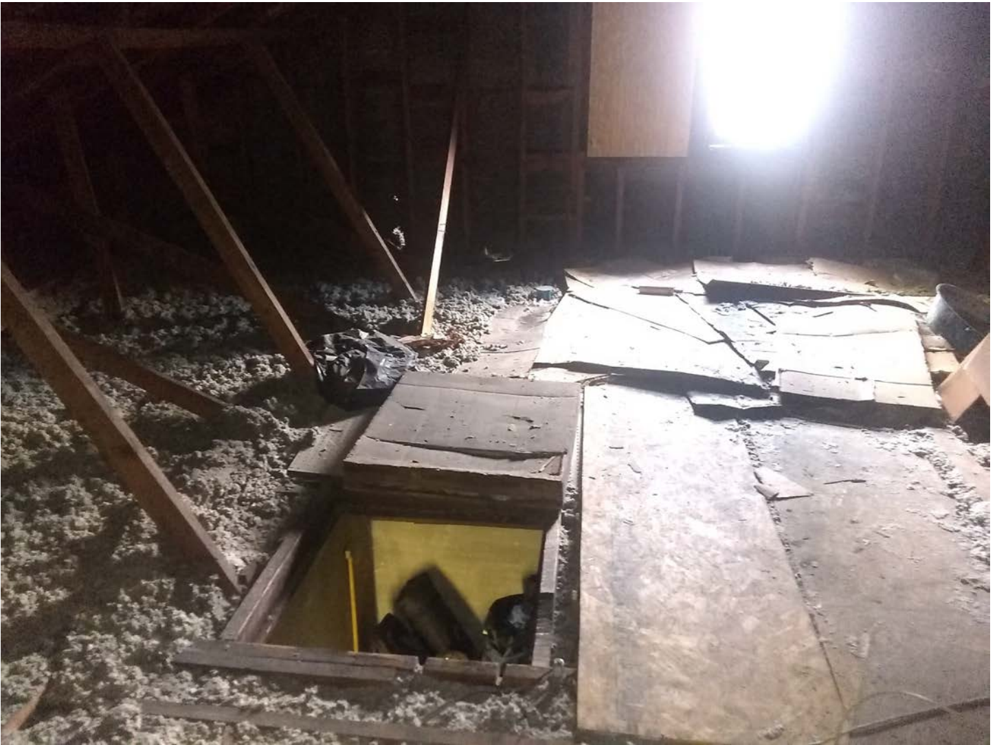
Proposed stairs and landing will run north-to-south in alignment with the access port photographed here.
