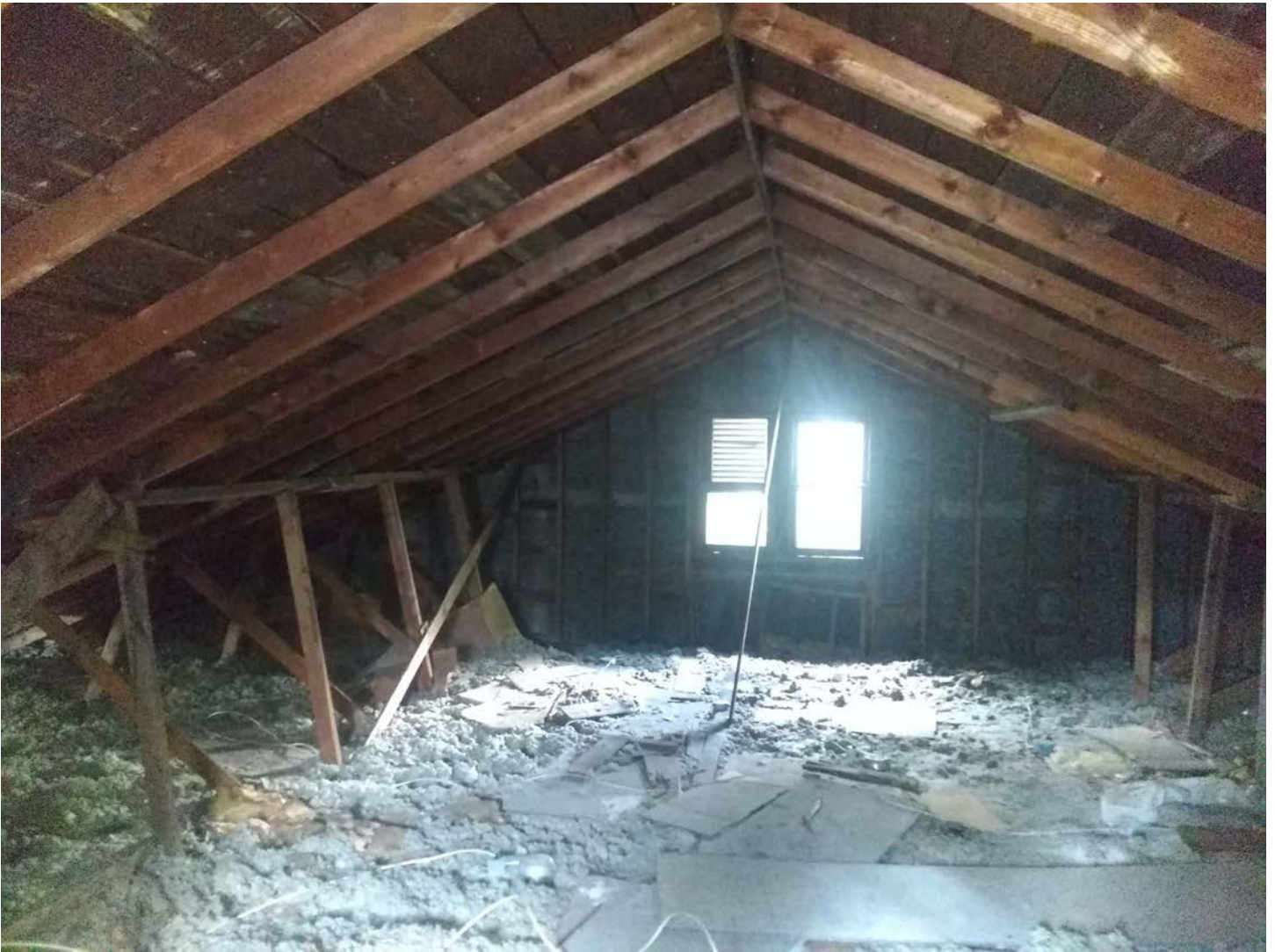
Facing north. View of proposed room and bath area. Note the left upper window was replaced with a louvered vent. This will be replaced with a newly fabricated matching window.
