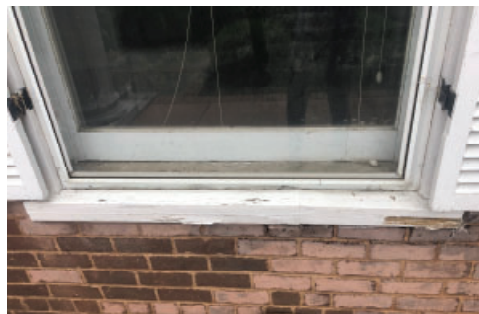
COMPROMISED WOOD (PINE) SILLS
