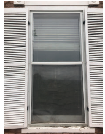
COMPROMISED WOOD (PINE) LOUVERED SHUTTERS
