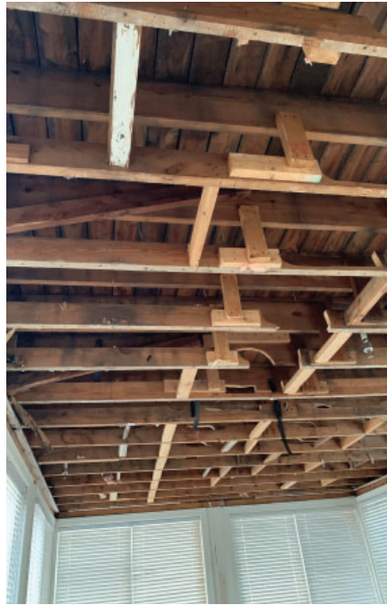
COMPROMISED PORCH STRUCTURE
