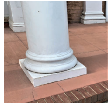
INCREASE PLINTH DEPTH 4" TO RAISE TORUS ABOVE NEW TENNESSEE MARBLE PAVERS ON EXISTING CONCRETE TERRACE
