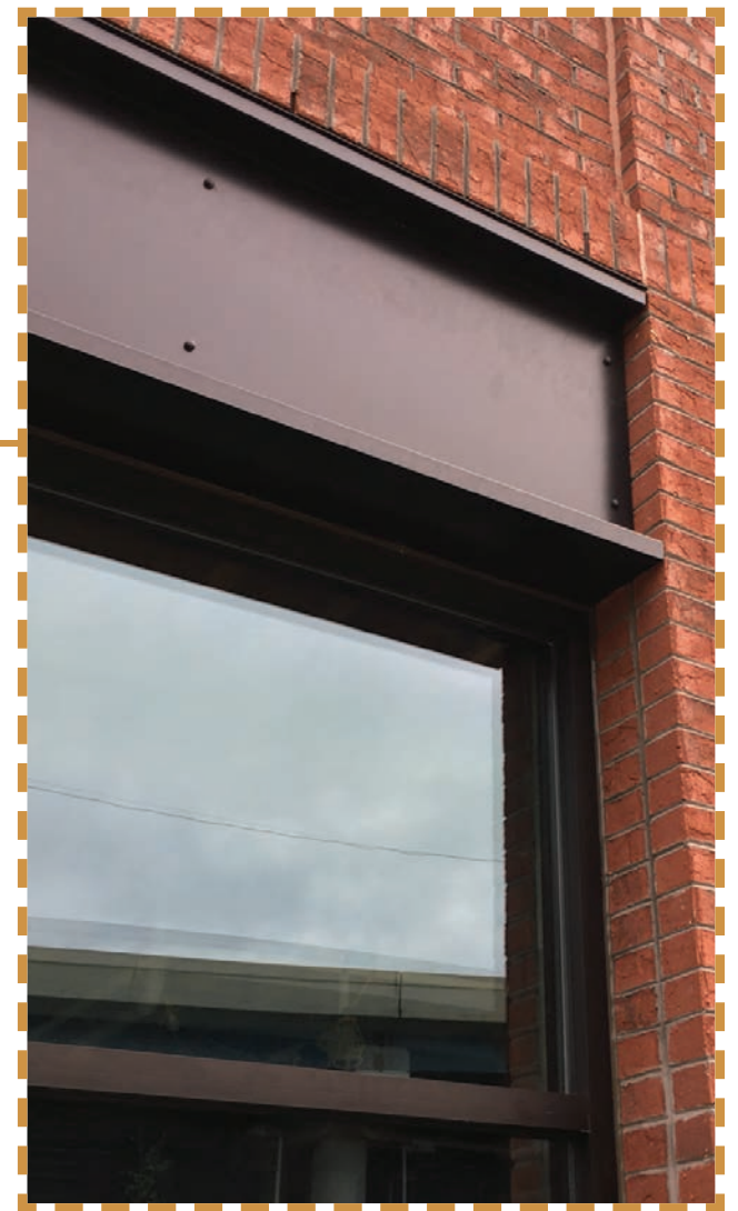
Similar Faux Steel Beam Condition
