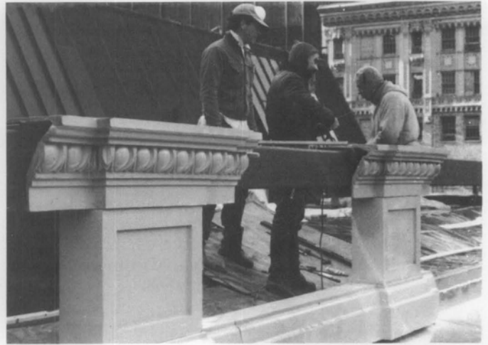
Illus. 18. Substitute materials must be properly installed to allow for expansion, contraction, and structural security. The new balustrade (a polymer concrete modified with glass fibers) at Carnegie Hall, New York City, was installed with steel structural supports to allow window-washing equipment to be suspended securely. In addition, the formulation of this predominantly epoxy material allowed for the natural expansion and contraction within the predesigned joints. Photo: Courtesy of MJM Studios.
