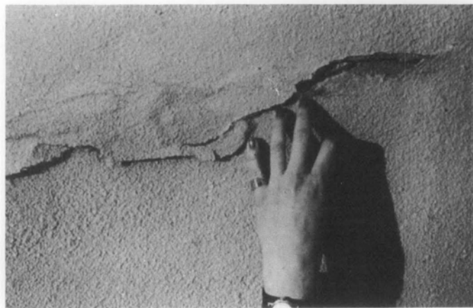
Illus. 6. Substitute materials should never be considered as a cosmetic cover-up for they can cause great physical damage and can alter the appearance of historic buildings. For example, a fiberglass coating was used at Ranchos de Taos, NM, in place of the historic adobe coating which had deteriorated. The waterproof coating sealed moisture in the walls and caused the spalling shown. It was subsequently removed and the walls were properly repaired with adobe. Photo: Lee H. Nelson, FAIA.
