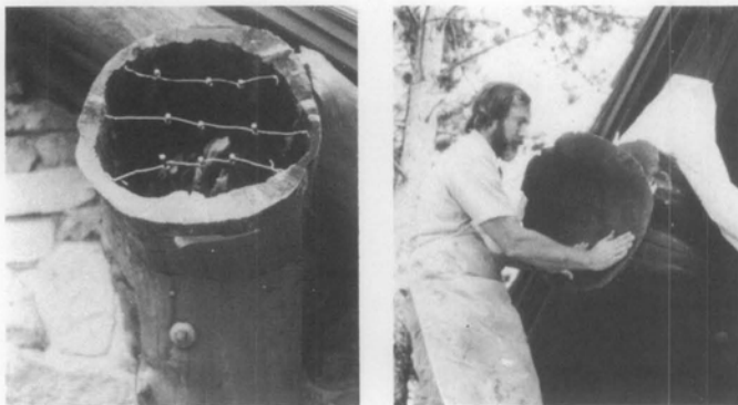
Illus. 17. Care must be taken to ensure that the replacement materials will work within a predesigned system. At the Norris Museum, Yellowstone National Park, the 12-inch diameter log rafters, part of an intricate truss system, had rotted at the inner core from the exposed ends back to a depth of 48 inches. The exterior wooden shells remained intact. Fiberglass rods (left photo) and specially formulated structural epoxy were used to fill the cleaned out cores and a cast epoxy wafer end with all the detail of the original wood graining was laminated onto the log end (right photo). This treatment preserved the original feature with a combination of repair and replacement using substitute materials as part of a well thought out system. Photos: Courtesy of Harrison Goodall.
