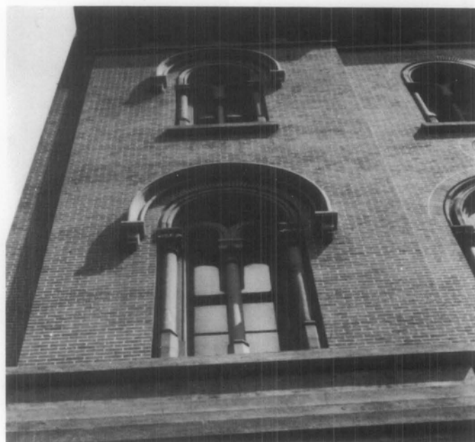
Illus. 8. Even when materials are not locally available, it may be possible and cost effective to find sources elsewhere. For example, the local sandstone was no longer available for the restoration of the New York Shakespeare Festival Public Theater. The deteriorated sandstone window hoods, were replaced with stone from Germany that closely matched the color and texture of the historic sandstone. Photo: John G. Waite.
