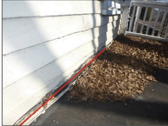
2.0 Picture 2 Areas of significant wood rot in the siding around the house
