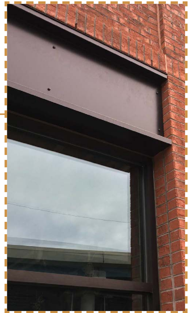
Similar Faux Steel Beam Condition
