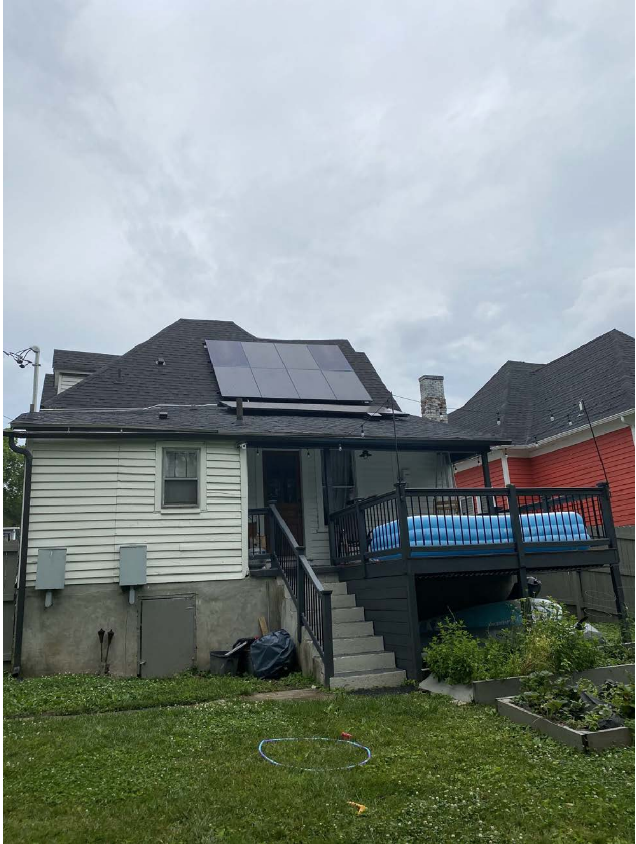
Documentation of current siding conditions.
