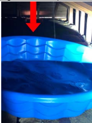
Plastic swimming pool appeared to be containment during leaking.
