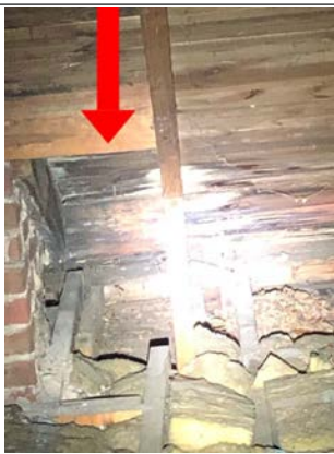
Example pics of sheathing / planking damaged noted in roofing section of report.
