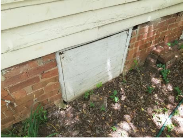
CRAWL SPACE DOOR TO BE REPLACED
