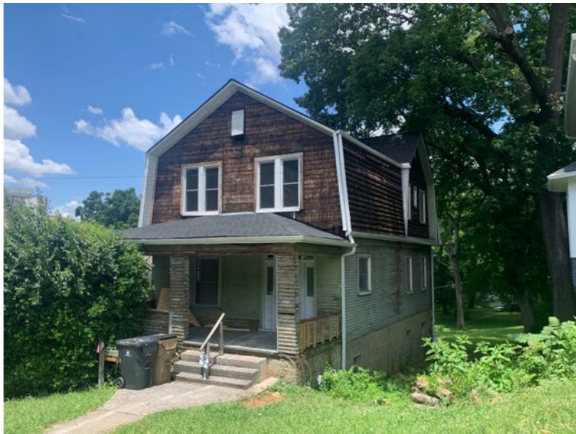
Fig. C, D, and E: 1404 Kenyon upon removal of vinyl siding from front (left) and rear (right), and southwest corner.
