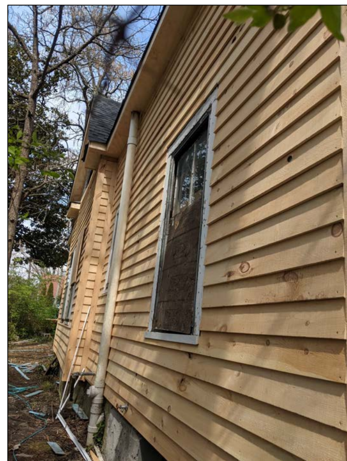
Inappropriate window trim with new siding
