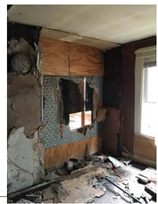
ROOTED AND TERMITE DAMAGE
