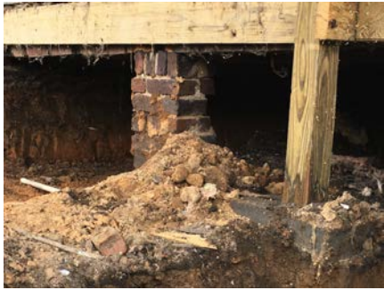
MOST OF DETERIORATED FOOTINGS REPLACED BY WOODEN POSTS
