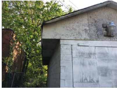
SUBSTANDARD GARAGE ADDITION
