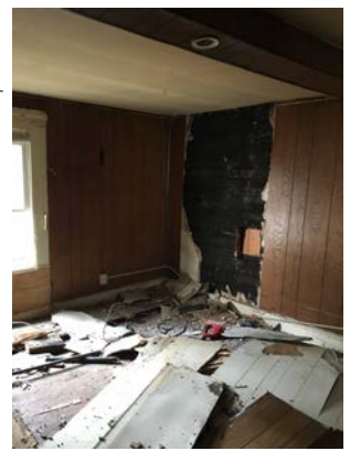
FIRE DAMAGE UNDER PANELING
