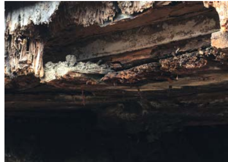
ROOT AND TERMITE DAMAGE
