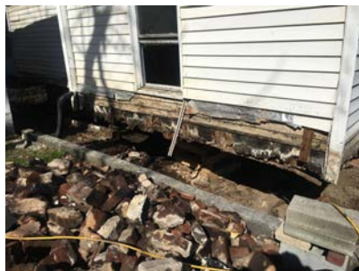
TERMITE DAMAGE UNDER VINYL SIDING
