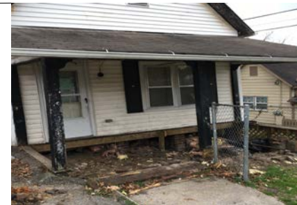
DETERIORATED FOOTINGS AT FRONT PORCH
