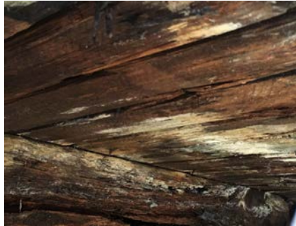
ROOT AND TERMITE DAMAGE
