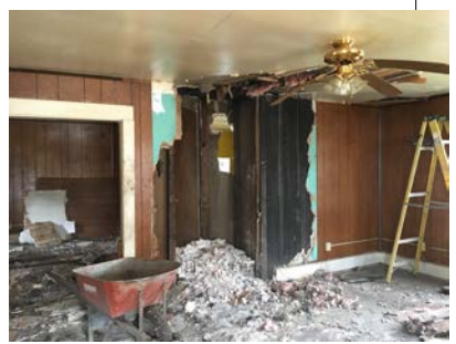
COLLAPSED FIRE BOX
