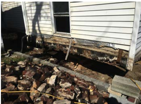
FOOTING CRUMBLER BY WATER DISCHARGE
