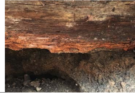
WEATHER DAMAGED DUE TO STRUCTURE SITTING DIRECTLY ON THE EARTH
