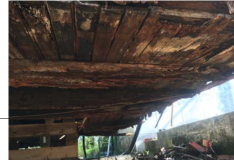
FLOOR SYSTEM DAMAGED BY ROOTS & MOLD
