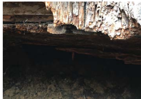
ROOT AND TERMITE DAMAGE
