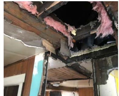
FIRE DAMAGE IN ATTIC
