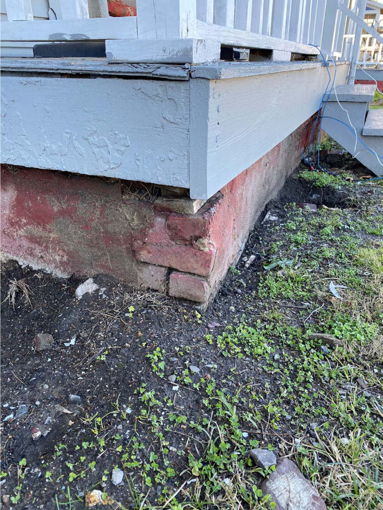
Front porch corner collapsing
