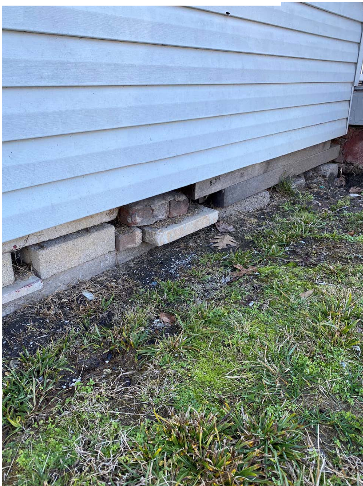
Front foundation collapsing (East) Supported by piecemeal brick and block
