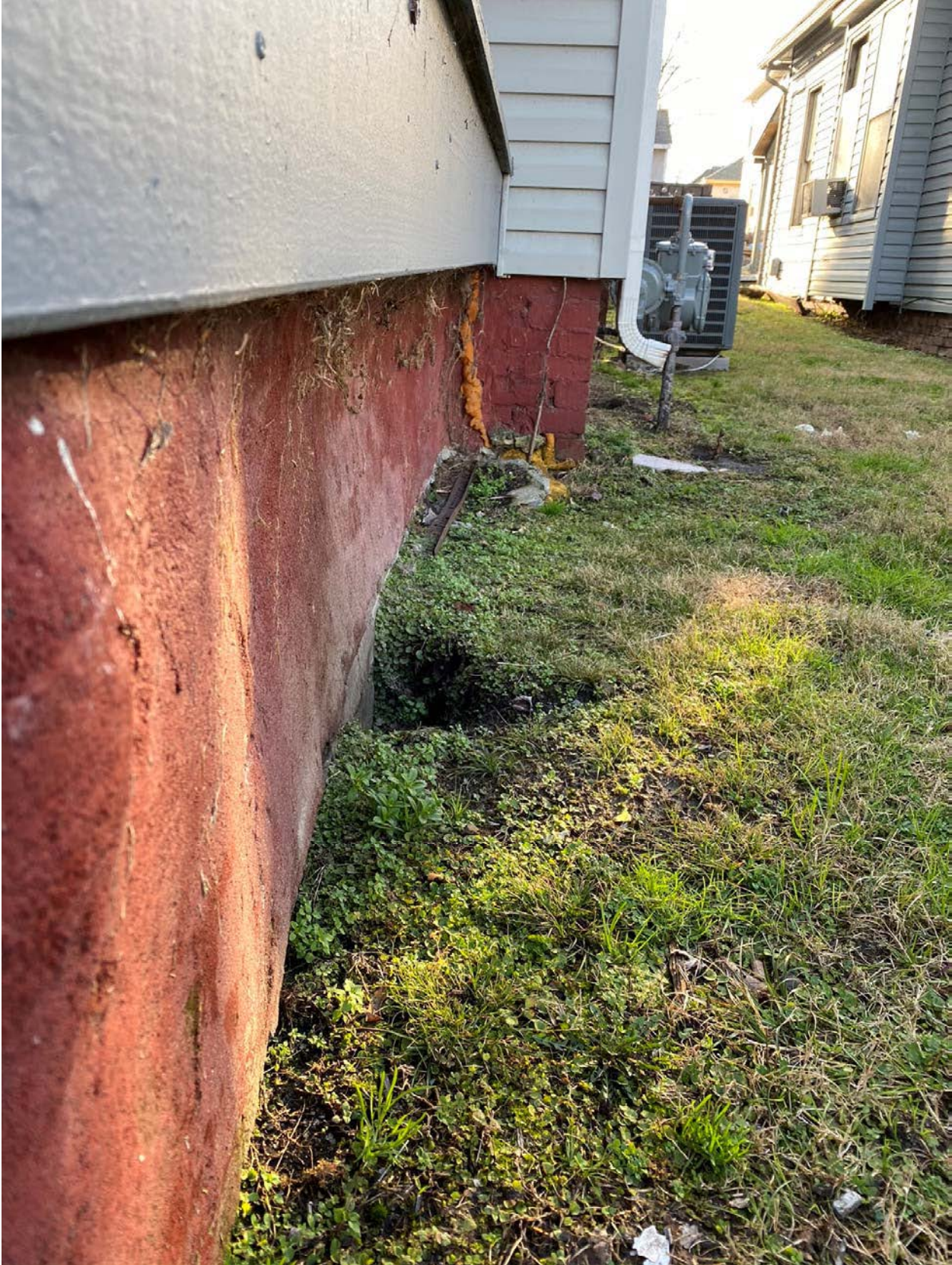
Front Porch brick caving in (North side)
