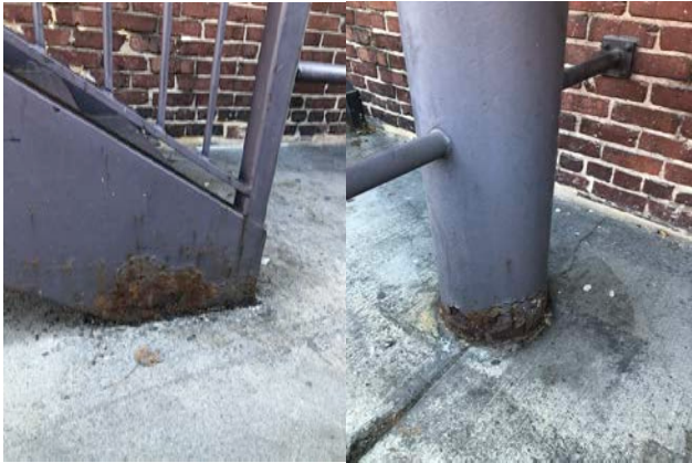
RUSTED METAL FIXTURES
