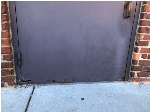
HOLES IN STAGE DOOR #1
