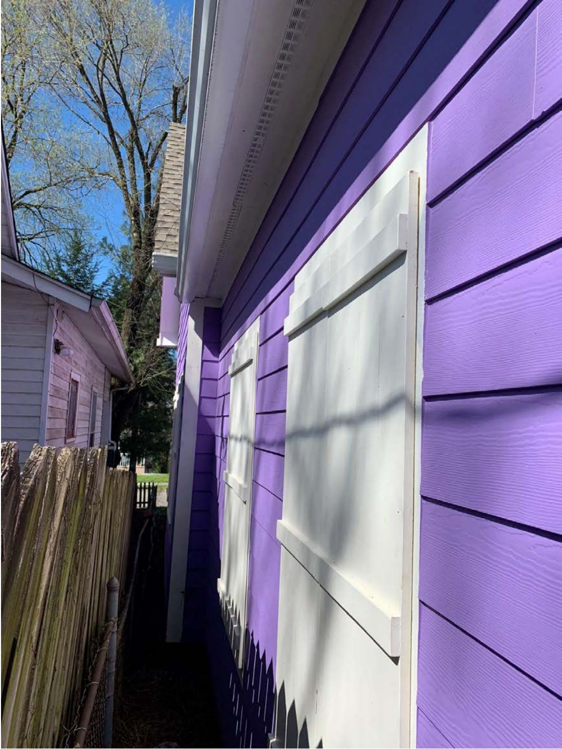
Window Covers where windows not allowed per building codes
