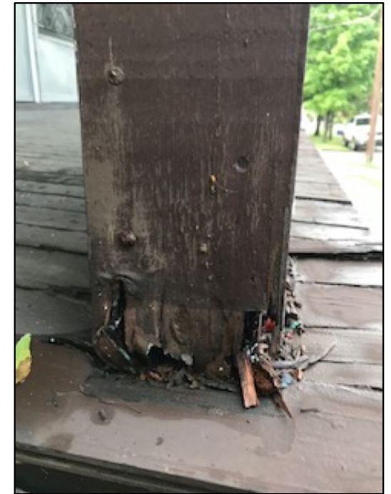
Deteriorated porch elements
