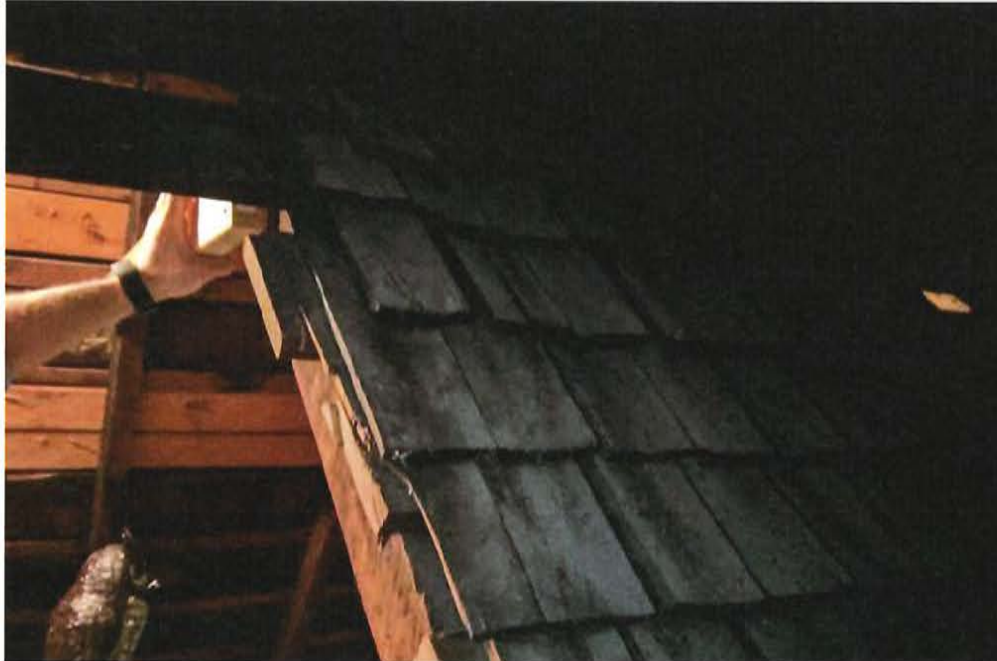
Wood shingle roof remaining inside of existing attic is evidence of major change to roofline in past. This section of the roof is the opposite side of the existing gabled section of the current roof. Best analysis of historic aerial photos leads to an estimate of change prior to 1935.
