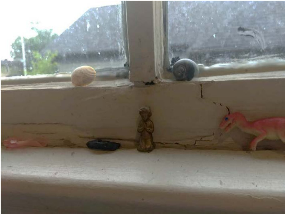
Photo showing condition of window rail, muntin, and catches.
