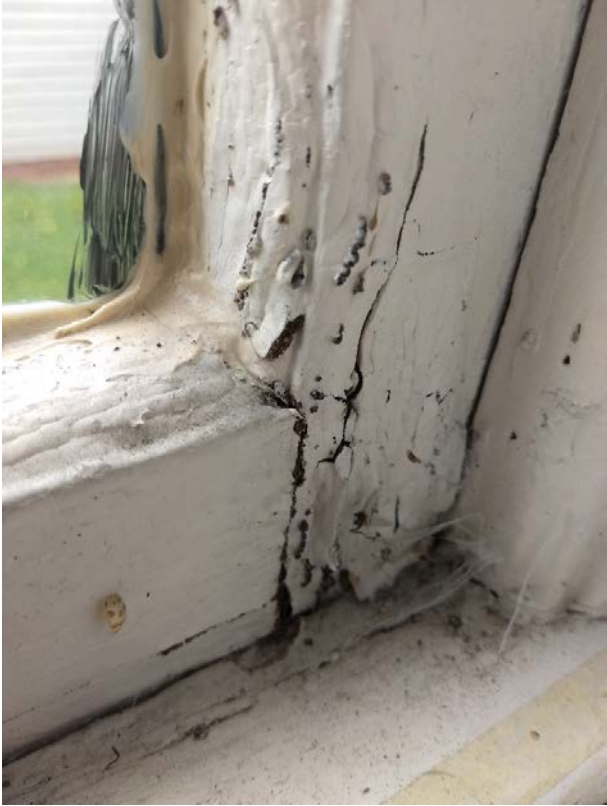
Photo showing condition of window rail and stile.
