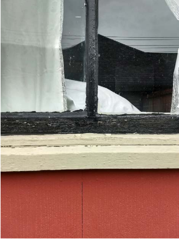
Photo showing condition of trim around windows on exterior.
