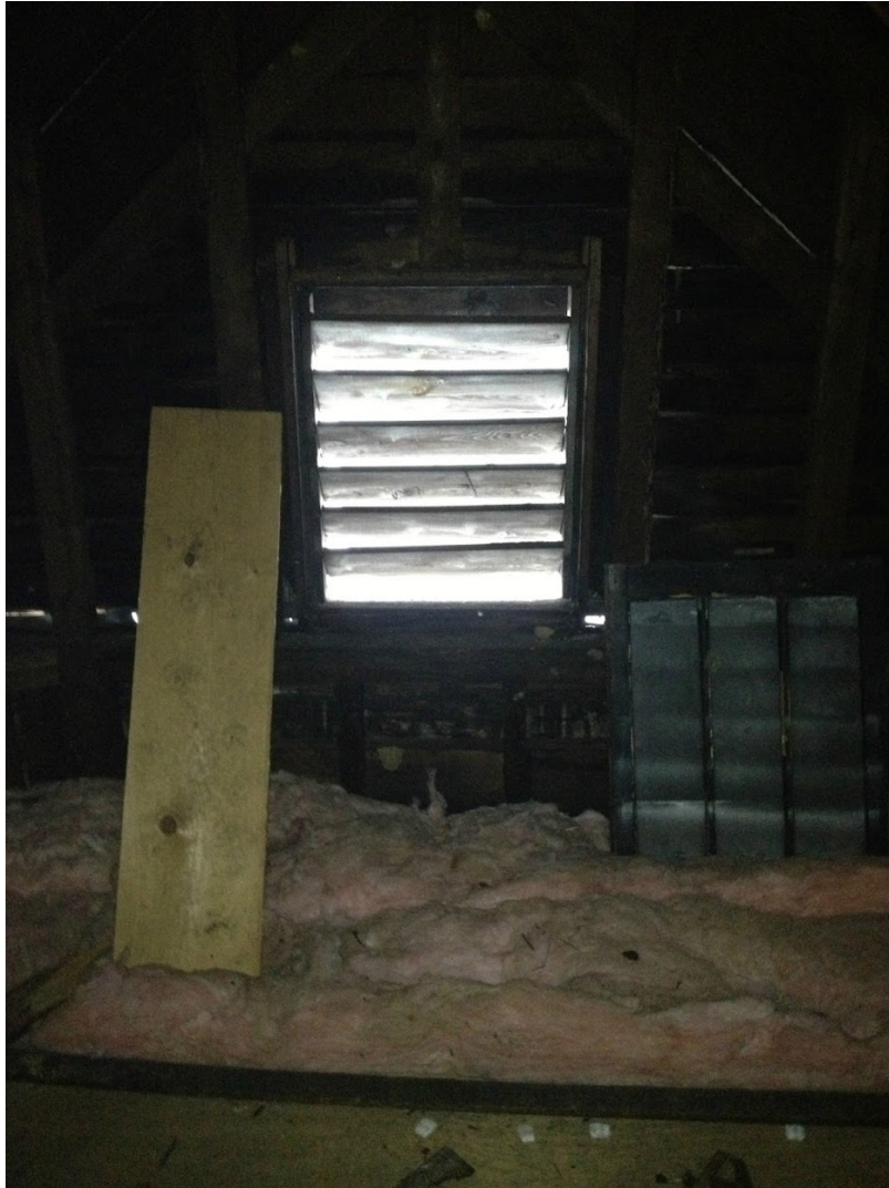
Gable vent that was originally a window. See photo above from previous owner with original window (now missing) on right. New casement window will have the same mullions.
