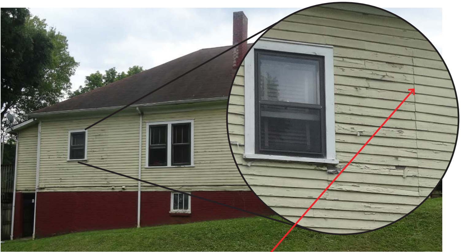
patch line in siding shows location of original double window to be restored
