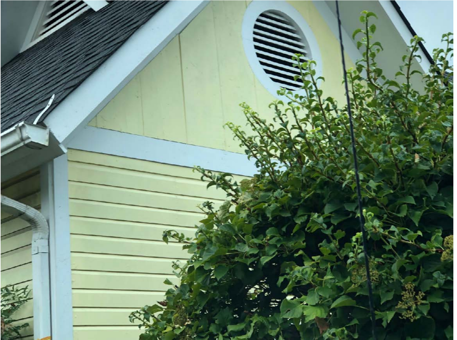
Vertical siding with texture on gable of accessory structure in same alley (photo provided by applicant)
