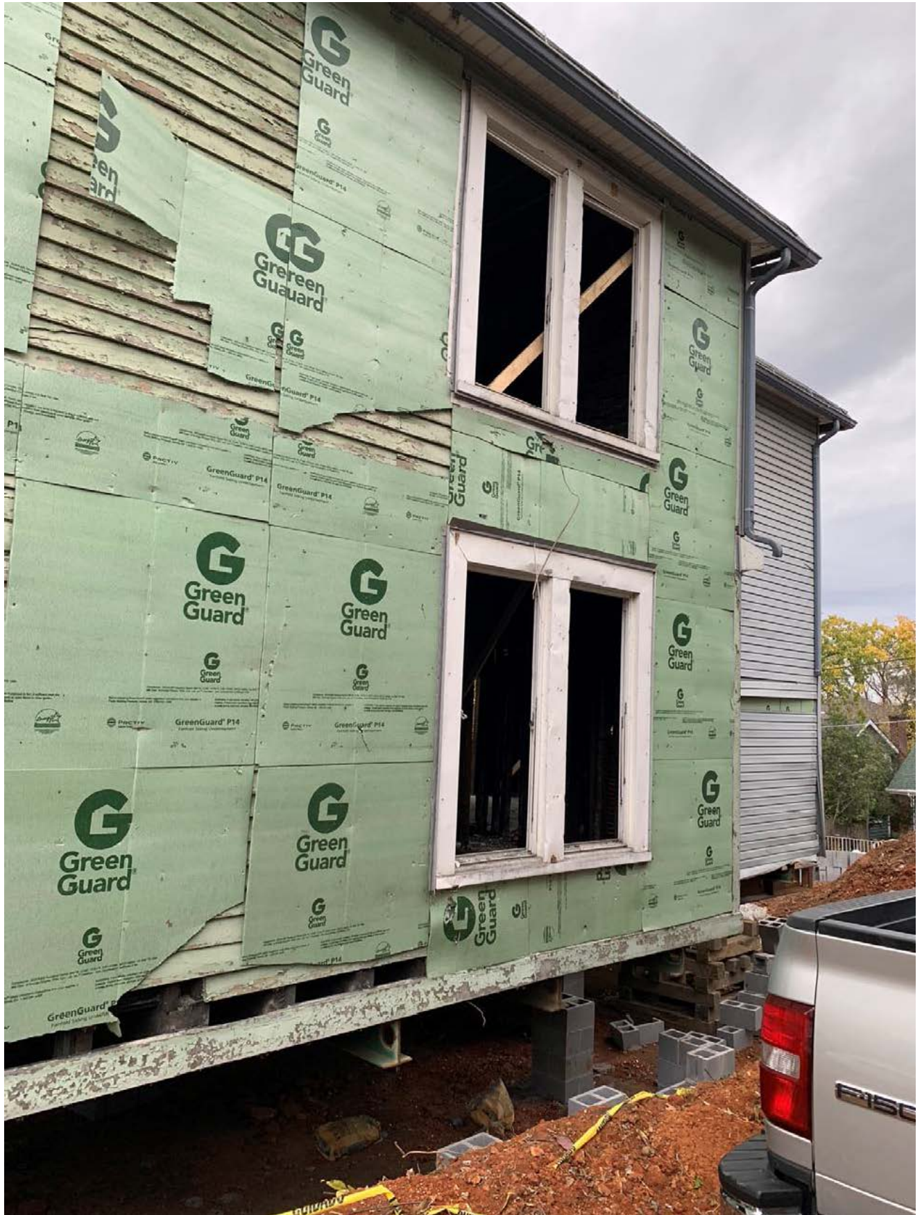
1717 Laurel Ave. -East façade looking north toward rear showing existing back recessed portion
