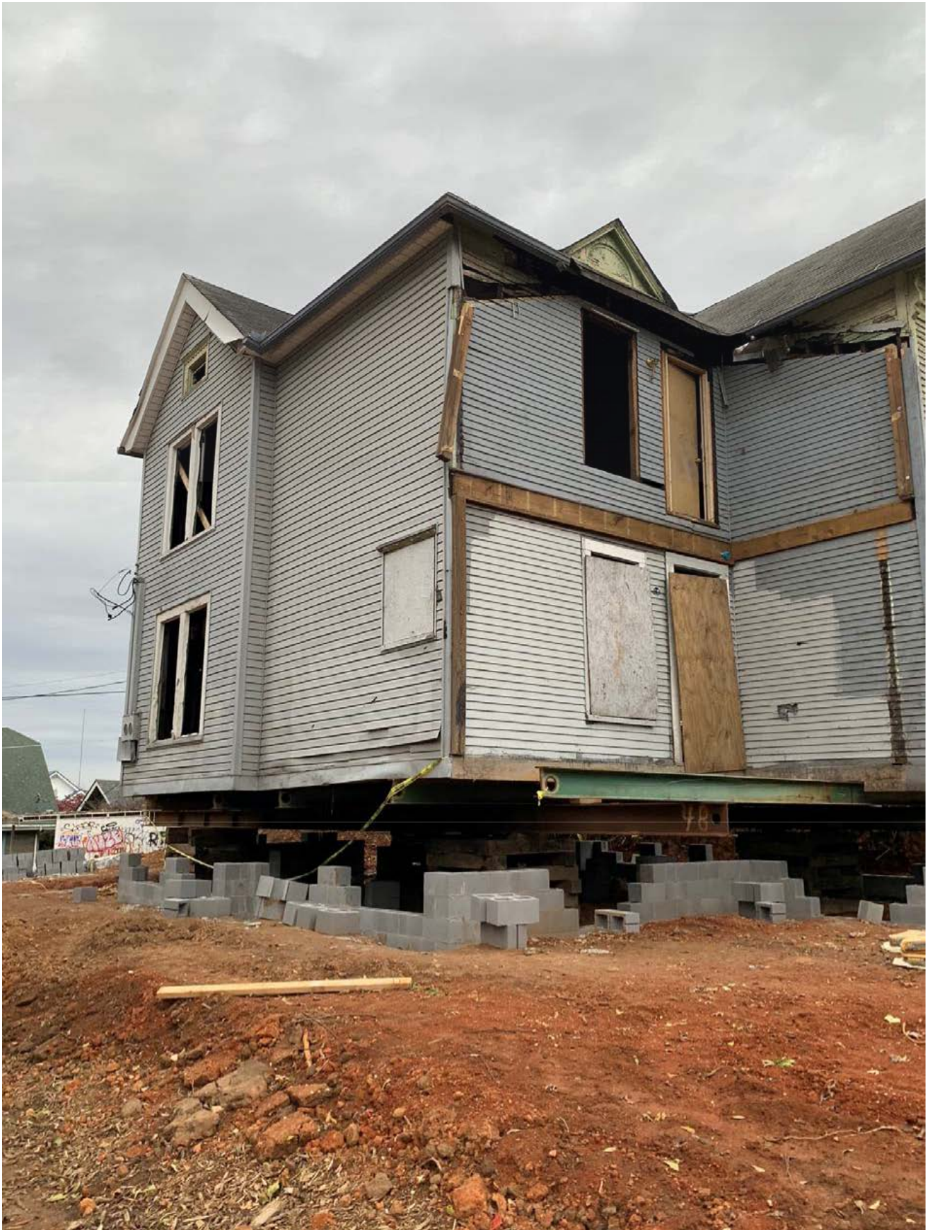
1717 Laurel Ave. - Front and west façades showing removed front porch looking northeast
