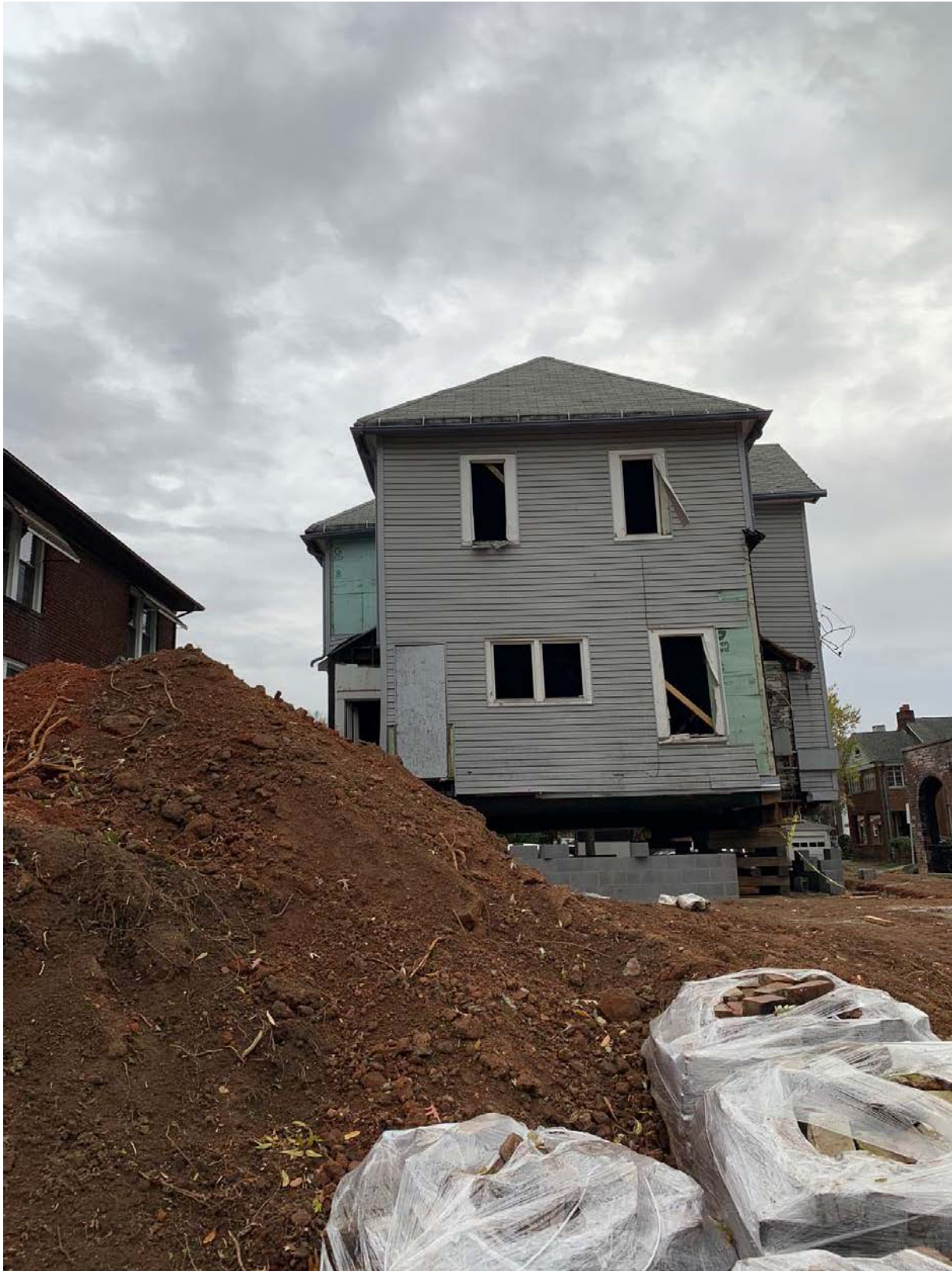
1717 Laurel Ave. - Rear (north) façade as viewed from back yard showing where the two 1-story additions on each side were removed and which are the locations of the two proposed 2-story additions.
