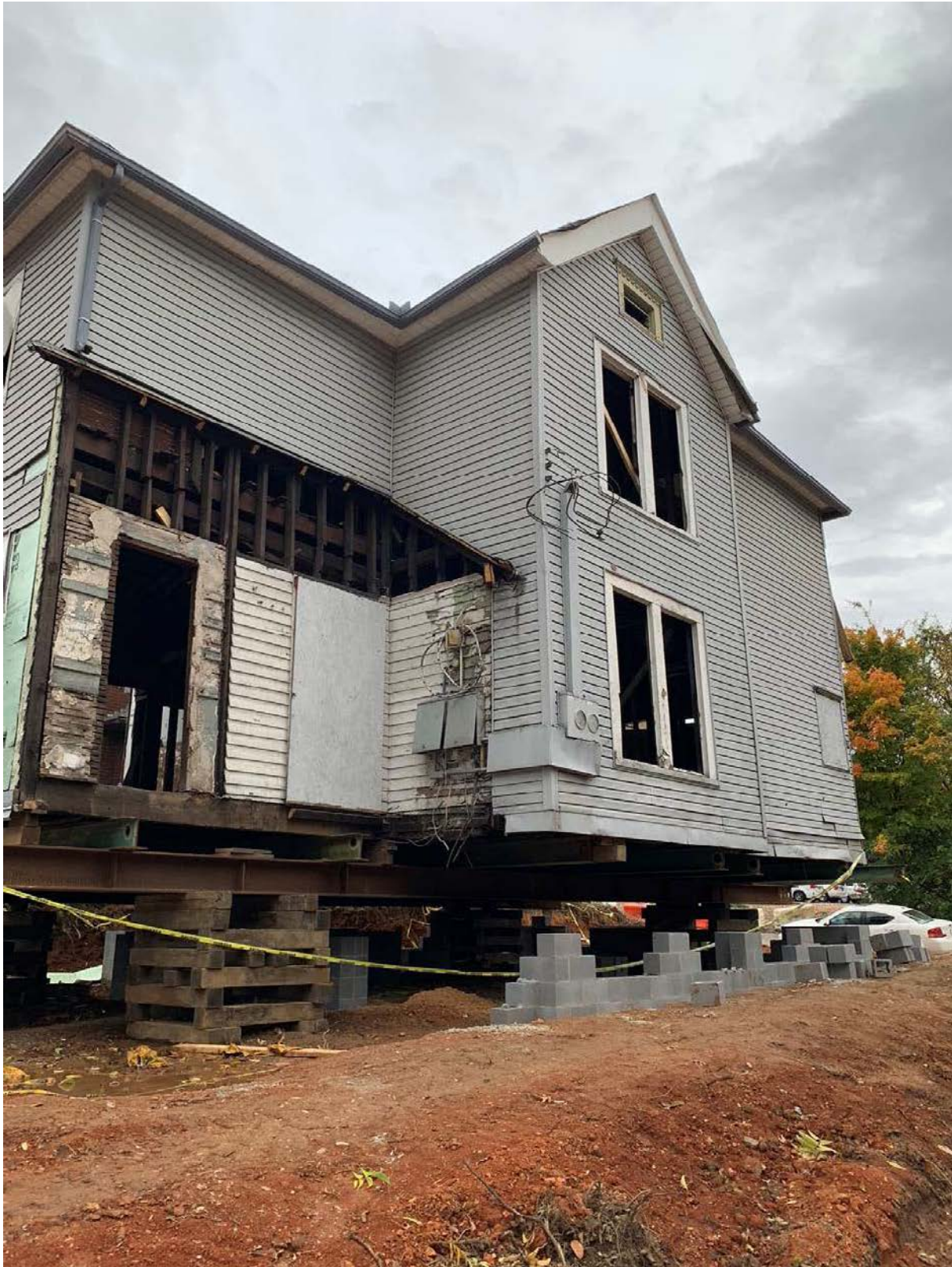
1717 Laurel Ave. - West side looking southeast. Rebuild former addition to two stories high. Add shed roof to differentiate. New shed roof location indicated by the orange line. 6" offset on right side, 1' on rear.
