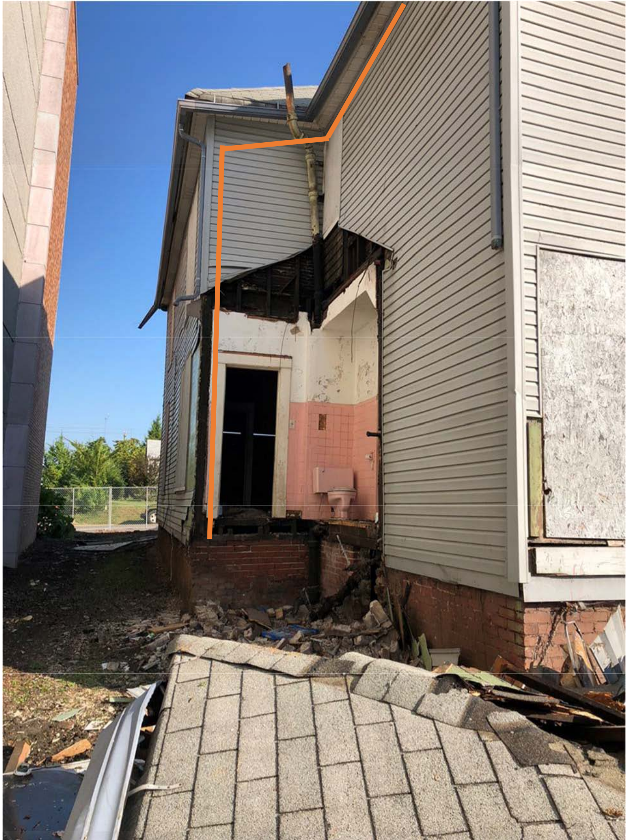
1810 Highland Ave. - Future east façade showing removed 1-story addition and location of proposed 2-story addition
