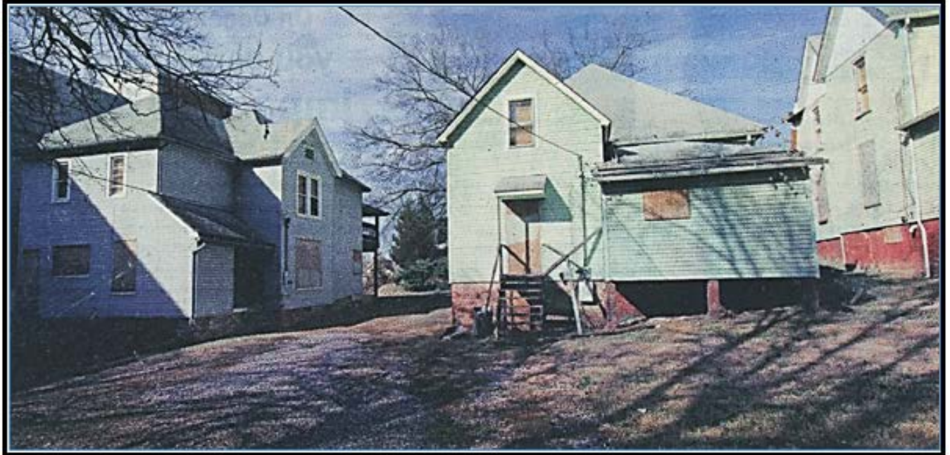
Rear of 1810 Highland Avenue (on left) before move showing pre-existing rear addition
