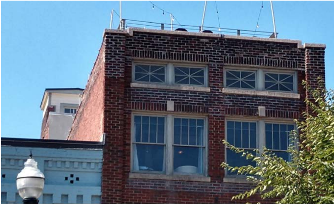
29 Market Square roof top guardrail – zoomed-in view from middle of Market Square
