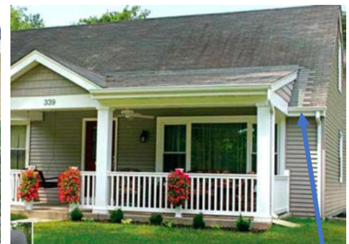
Example of the area beneath the slope on each side of the shed roof infilled with painted wood siding.
