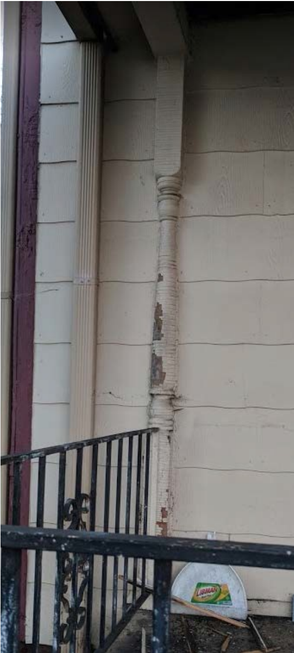
Existing embedded post at 401 Oklahoma:
