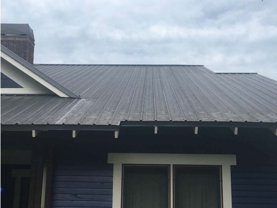
Metal Roofs on East Oklahoma Homes Using Non-Standing Seam, Exposed Hardware (e.g. like Tuff-Rib)
