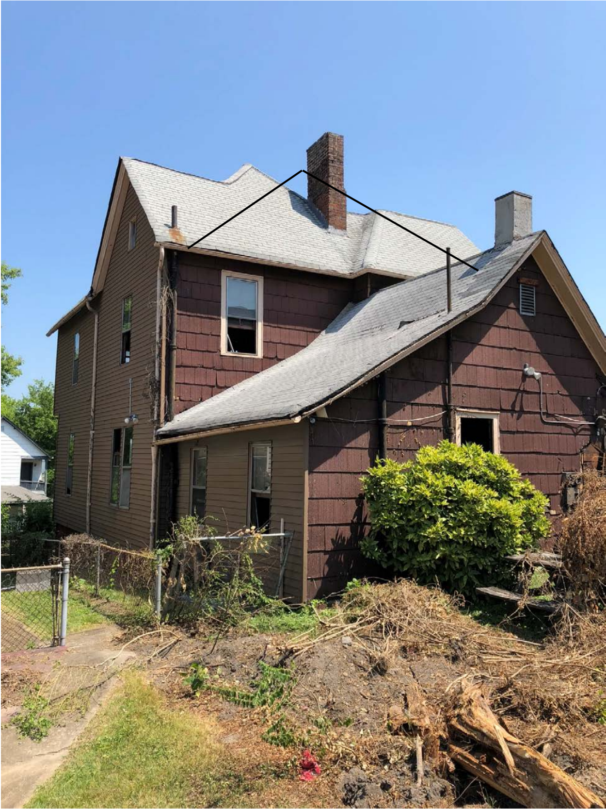
Back and West Side View showing roof line and addition to be demolished
