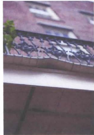
Buckling Wood T&G Balcony in the French Quarter.
