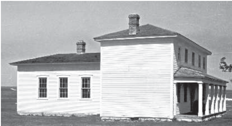
In a project at Fort Hays, Kansas, the wood frame officers' quarters were restored to the late 1860s--their period of significance. This included replacing a missing kitchen ell, chimneys, porch columns, and cornice, as well as closing a later window opening in the main block. The building and others in the museum complex is used to interpret frontier history. Photo: NPS files.
