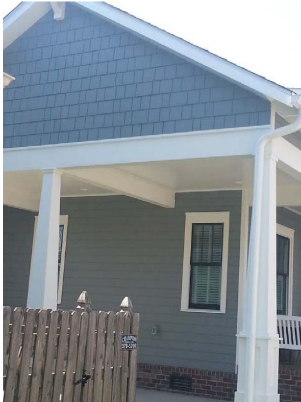
809 Eleanor - photo of fiber cement shingles installed in front gable at 817 Deery (new construction)
