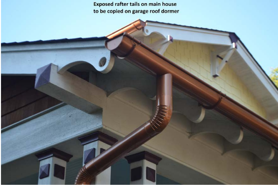
1012 Oak Ave – Rafter tails
