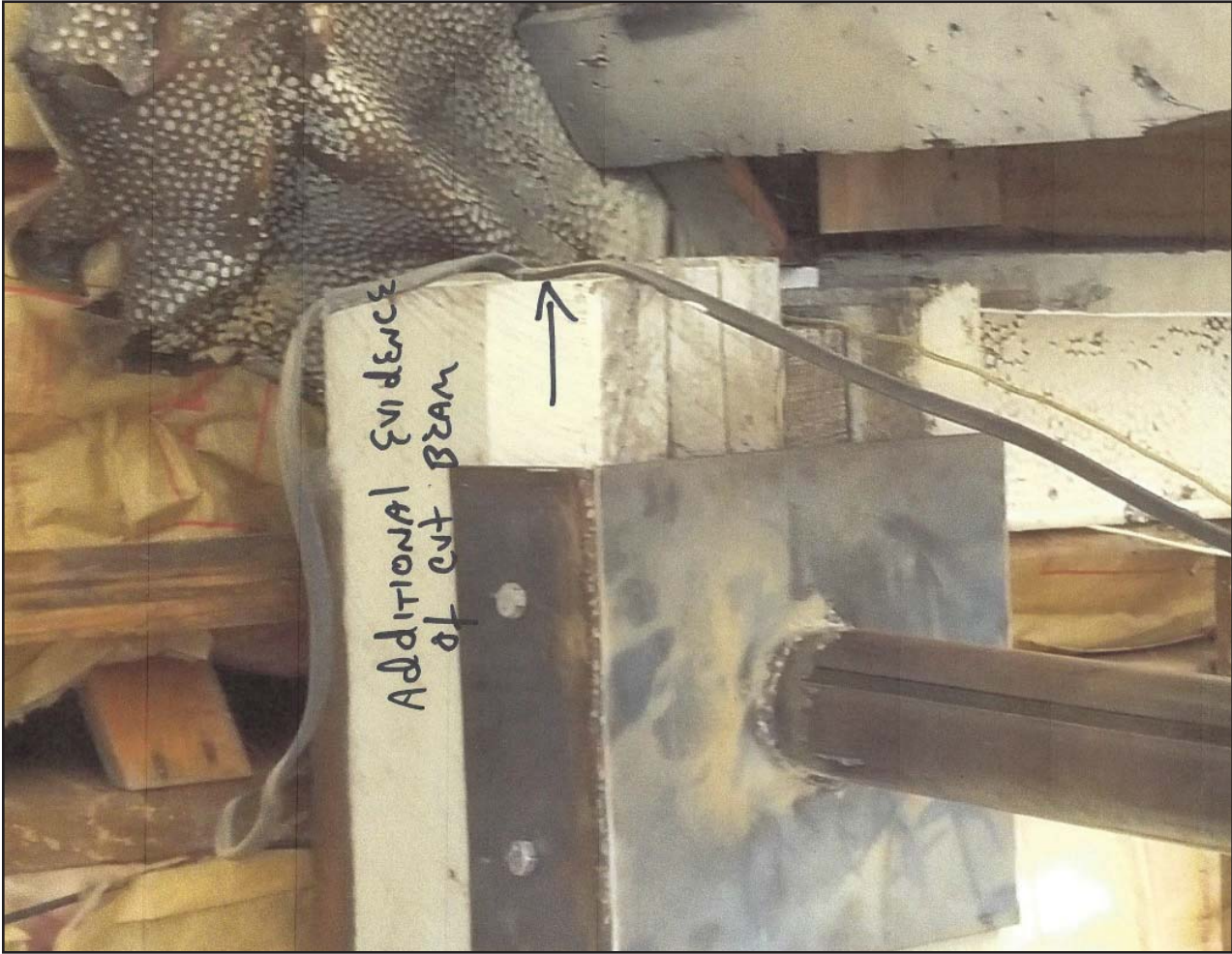
Additional evidence of cut beam
