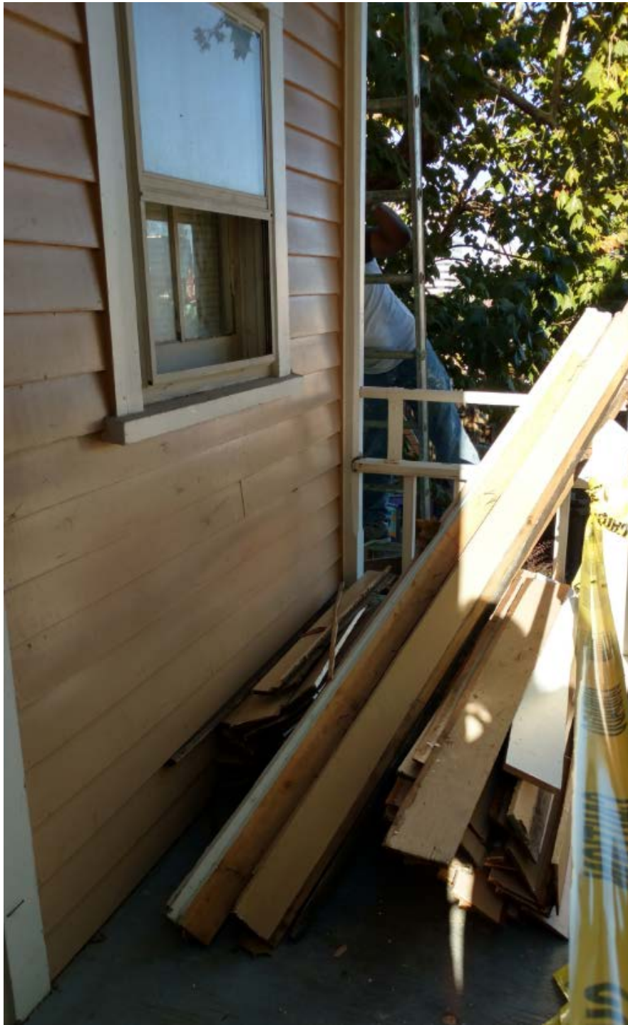
Rear of 404 11 th showing cut-away porch with new bathroom wall and window
