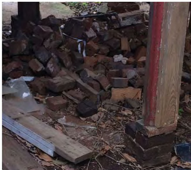
Original brick supports show us the dimensions of the original rear porches.
