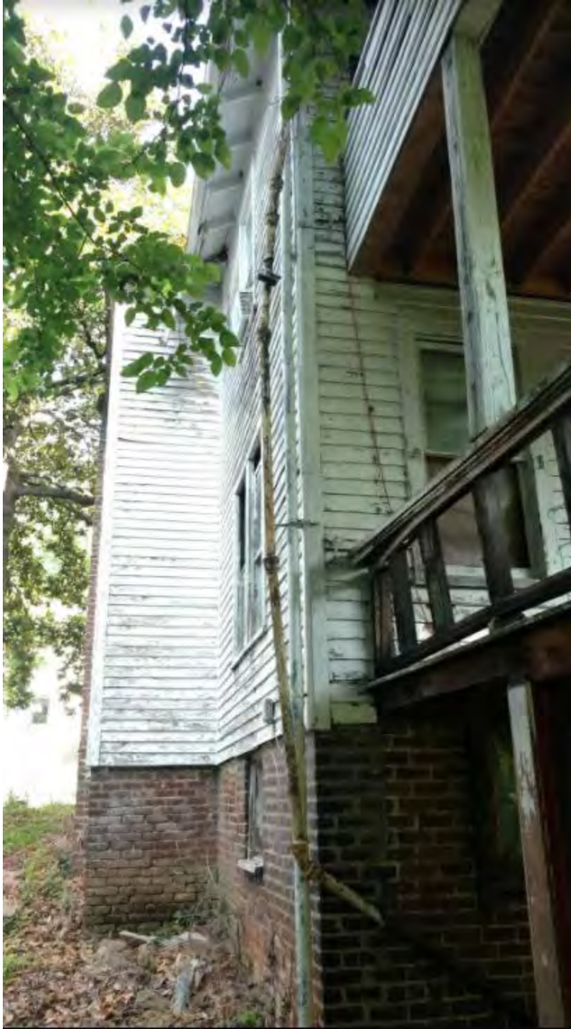
1424 Fremont - View of south side from rear showing tie-in of existing decks
