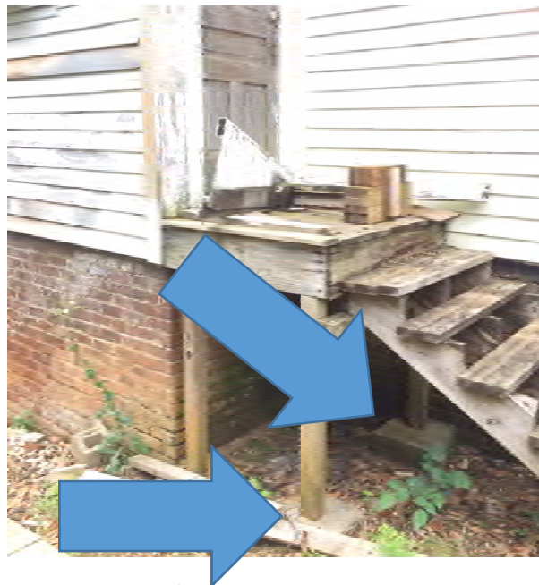
Cinderblock foundations to the makeshift landing also supports that there was never a wraparound porch.
