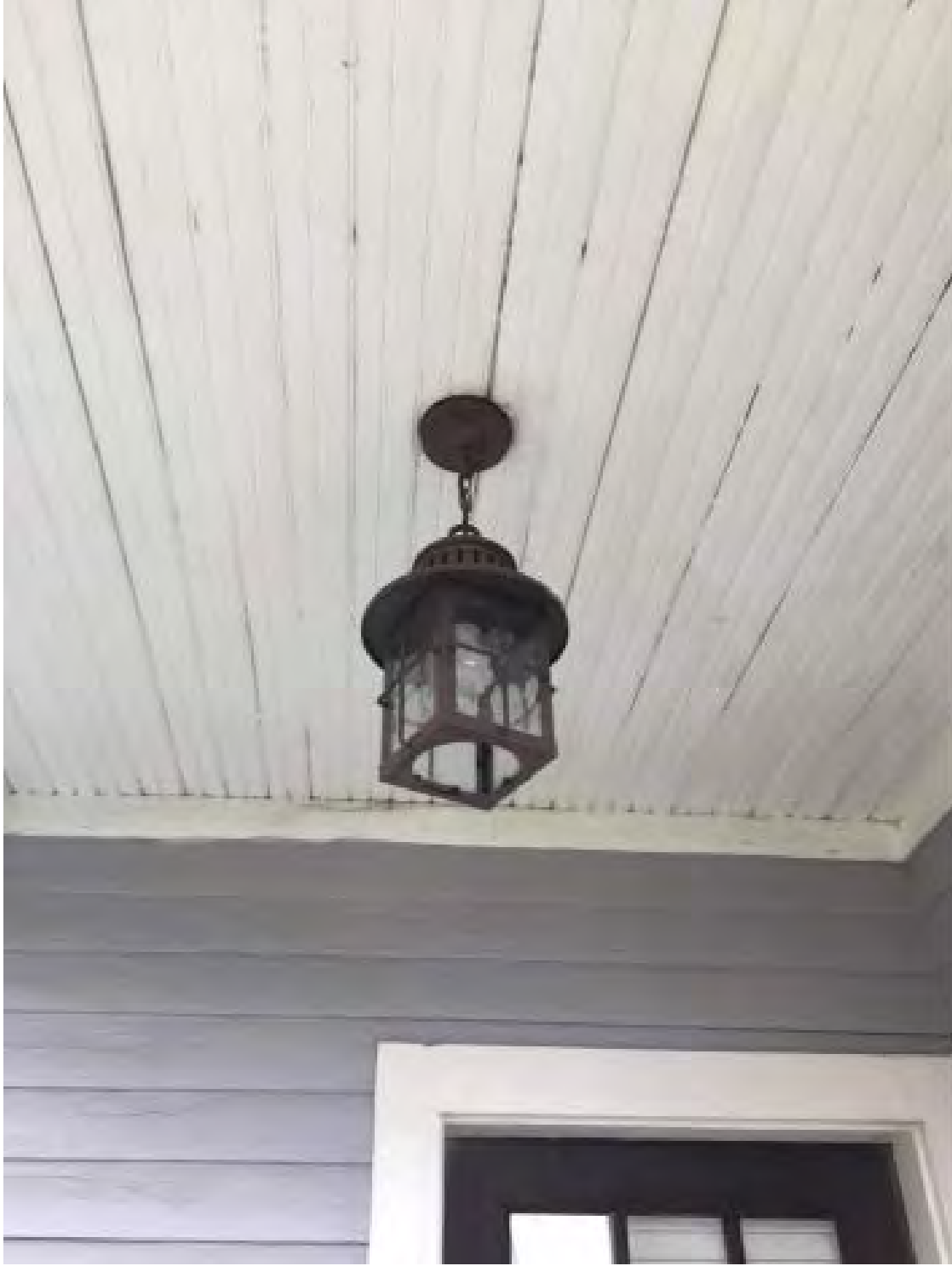
Beadboard-style tongue-and-groove on front porch ceiling to be matched as siding above the roof of the side room addition.
