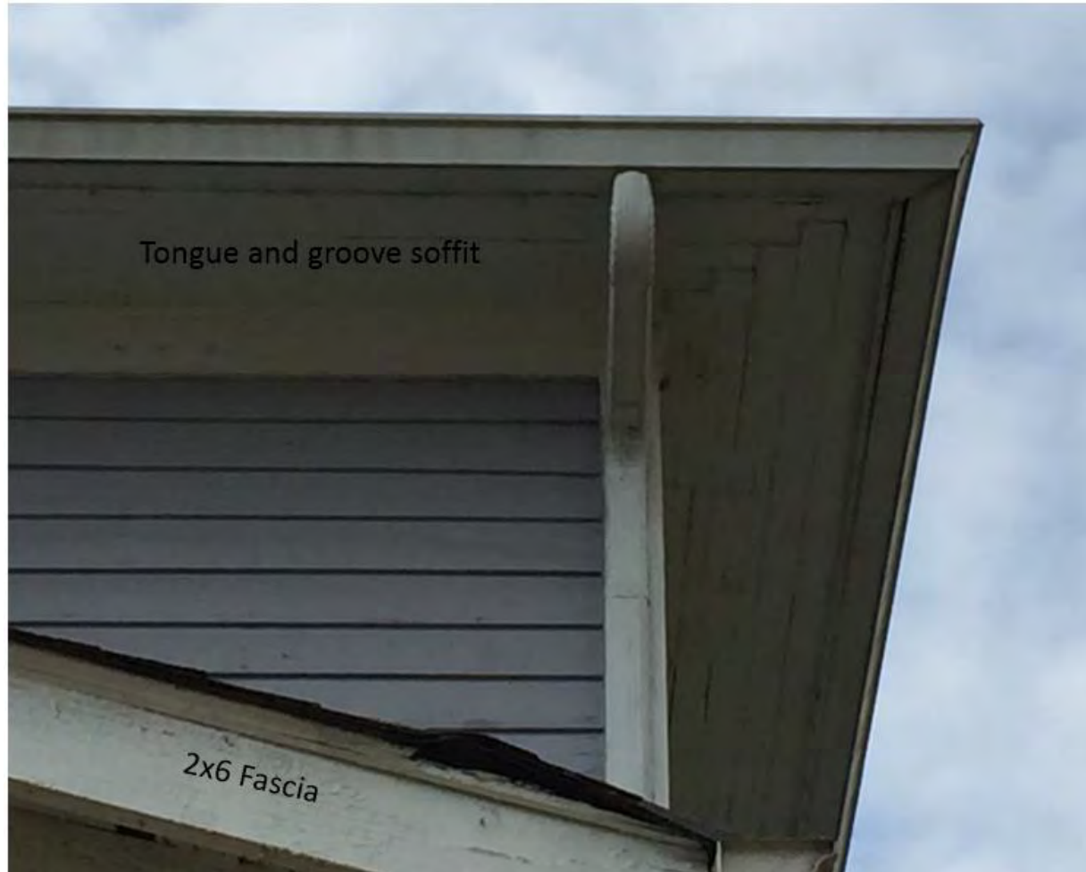
(Image 3) – Example of existing tongue and groove soffit and 2x6 fascia board on the Northeast side of the house (front).
