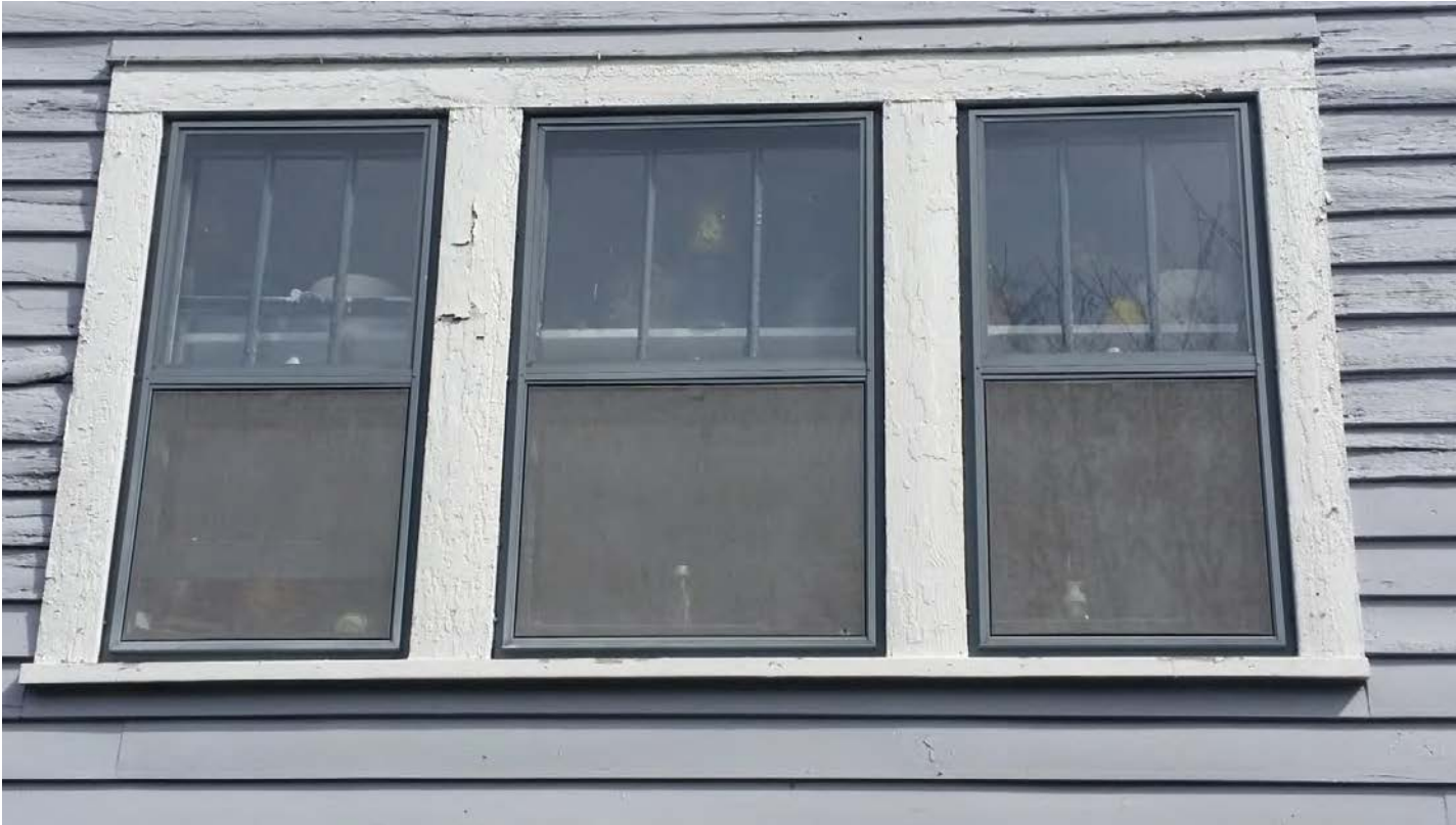
(Image 1) – Existing house windows in the kitchen on the West side of the house.
