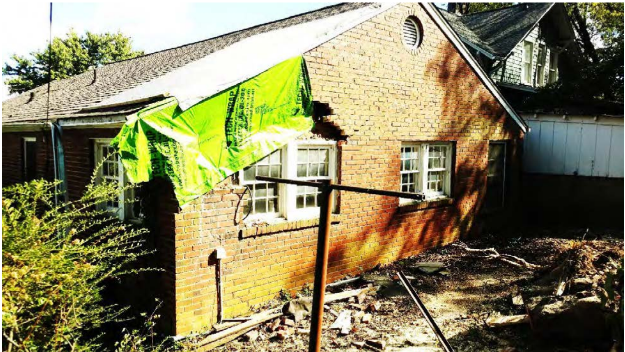
1115 Gratz Street – Rear facade showing damage
