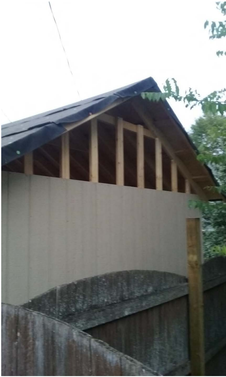
725 Deery - View of shed from southeast side -next to side yard fence
