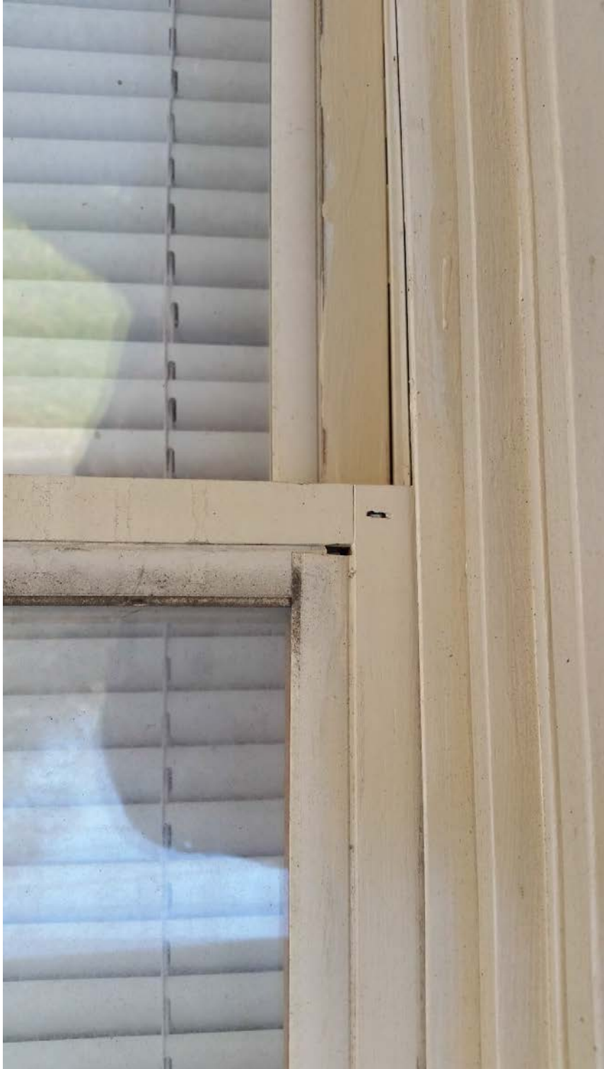
1400 Grainger Ave. – Non-historic front window to be replaced
