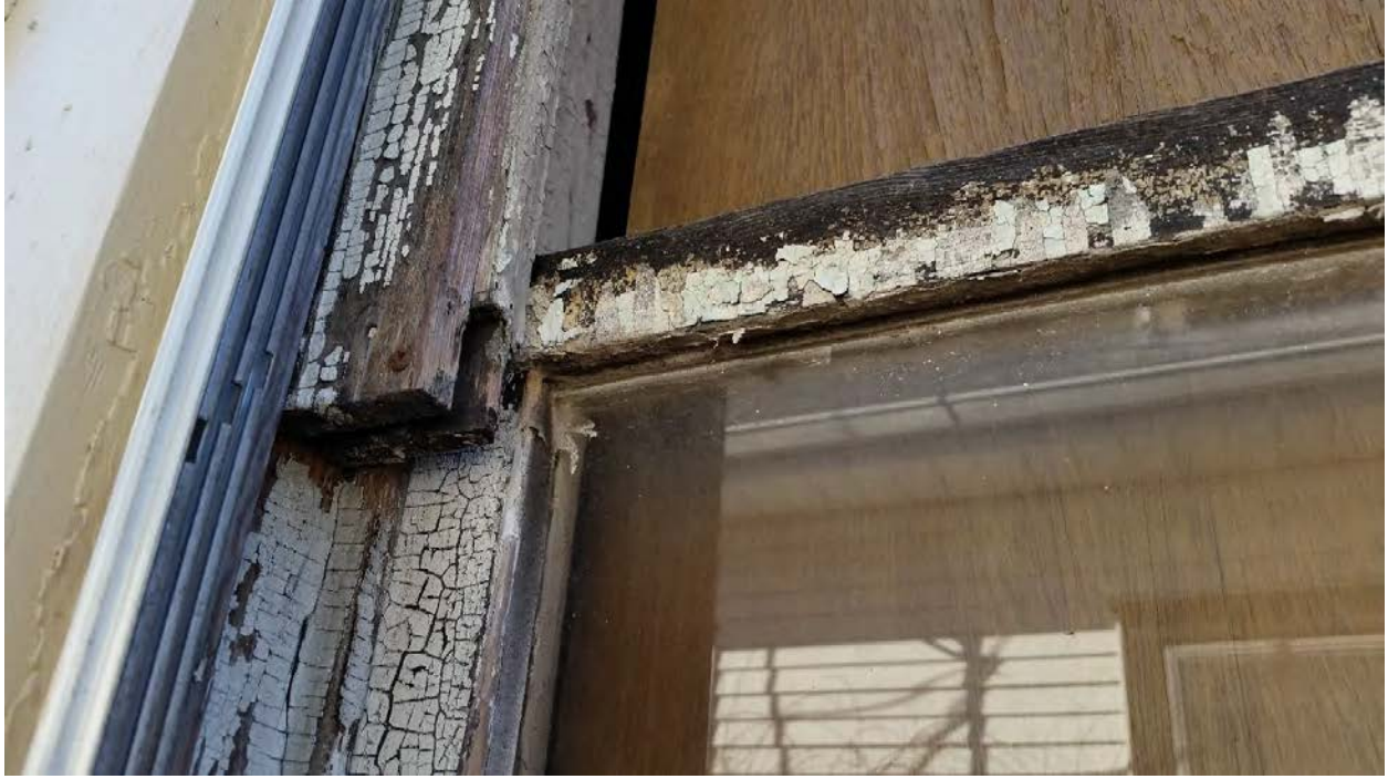
1400 Grainger Ave. – Detail of original of east side window to be replaced
