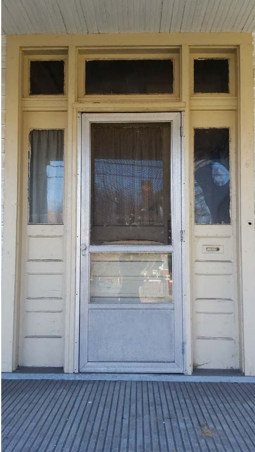
1400 Grainger Ave. – Front door to be repaired
