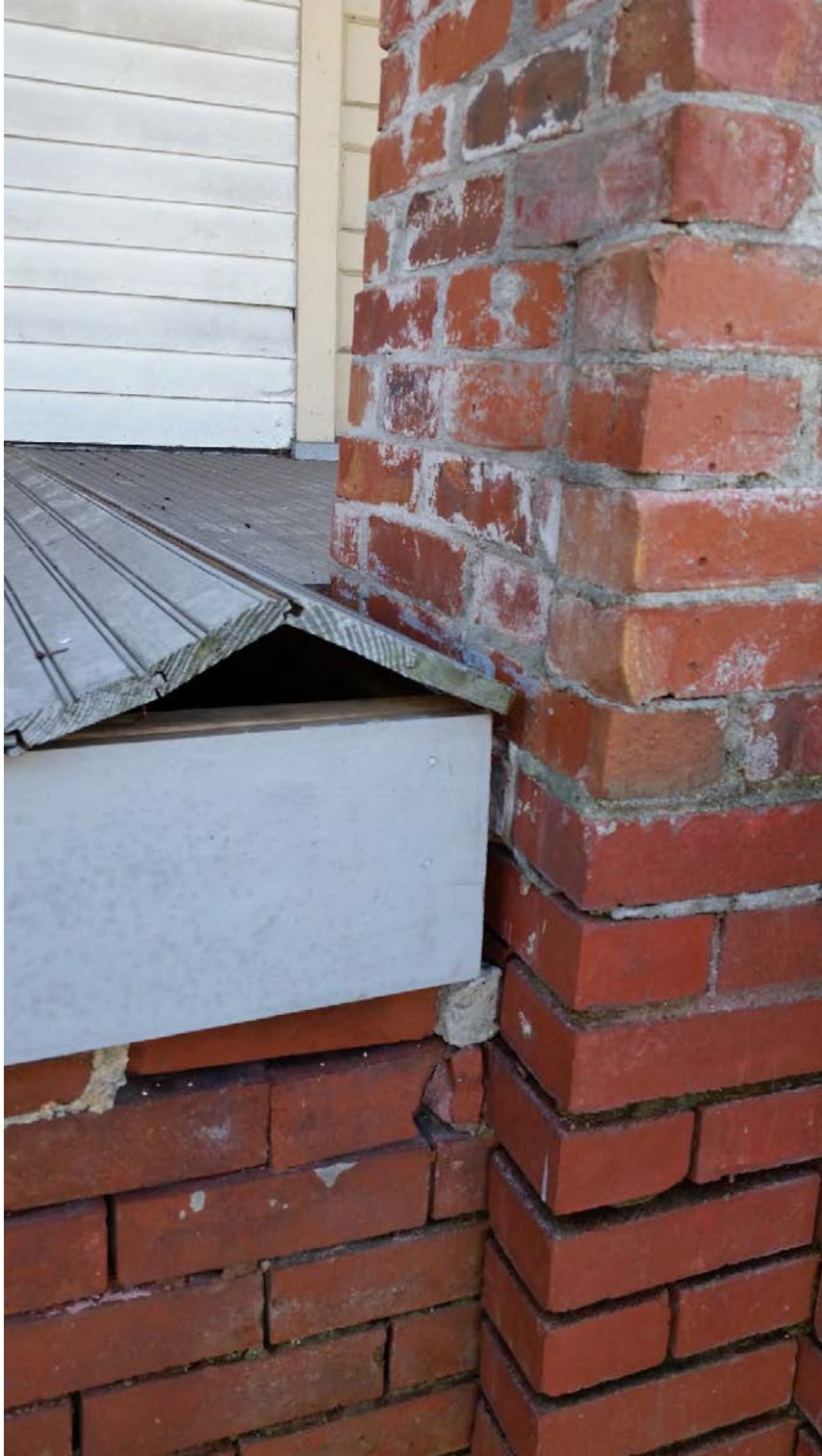
1400 Grainger Ave. - Porch support bases to be repointed and painted
